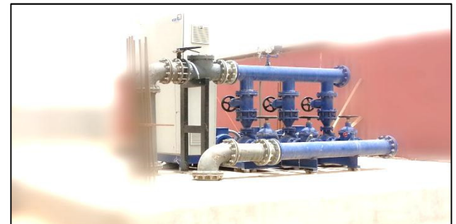
Transfer (Booster) Pumps
