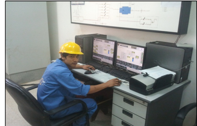
Modern Monitoring & Control Equipment
