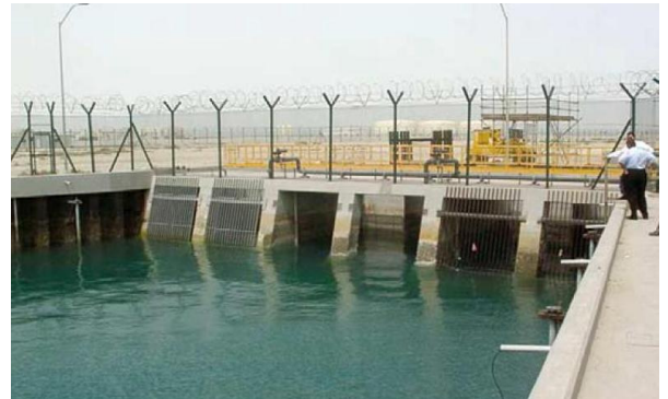
Outlet weirs (COWI Marine and coastal engineering)
