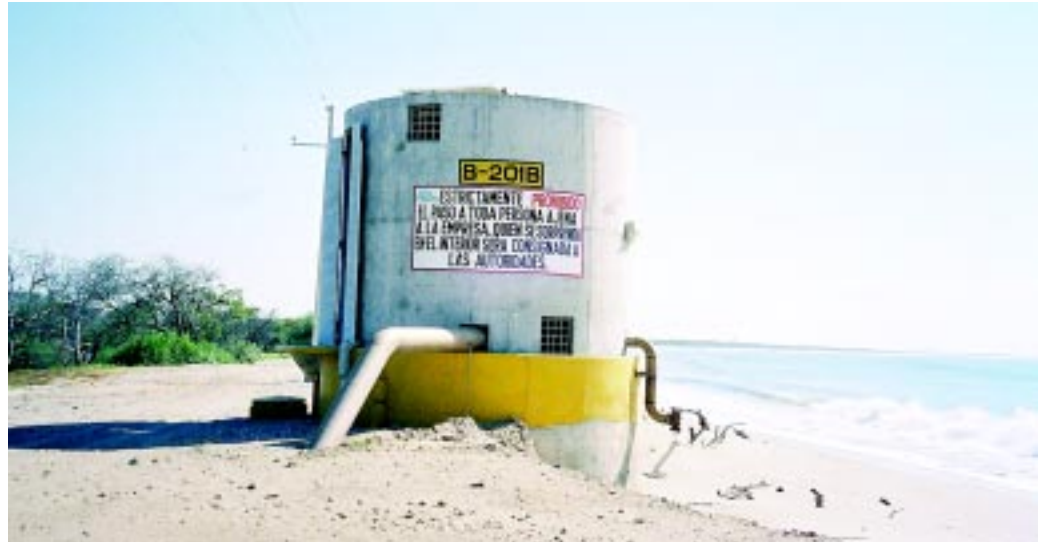
Figure 2 – Intake Beach Well of Large Seawater Desalination Plant
