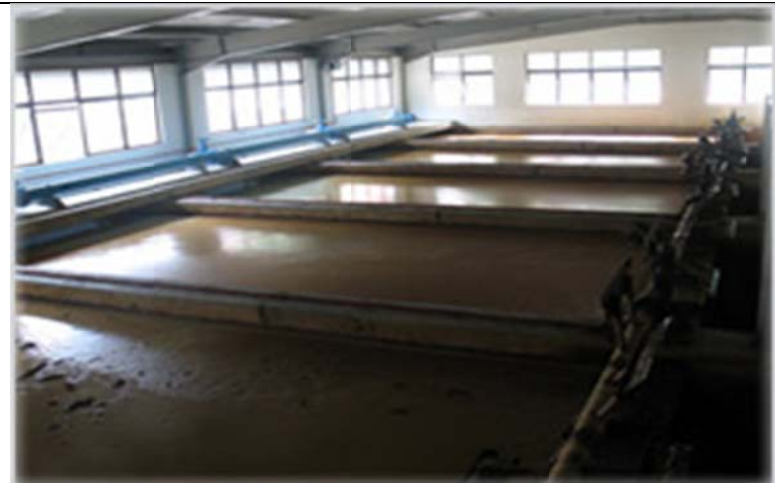
DAF Unit Floatation Tank (Thick Sludge Blanket on Top of Water being Skimmed by Skimmers/Scrapers)
