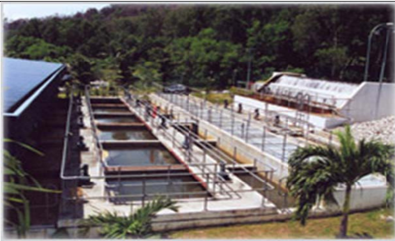
Overview of a DAF Unit for Water Filtration
