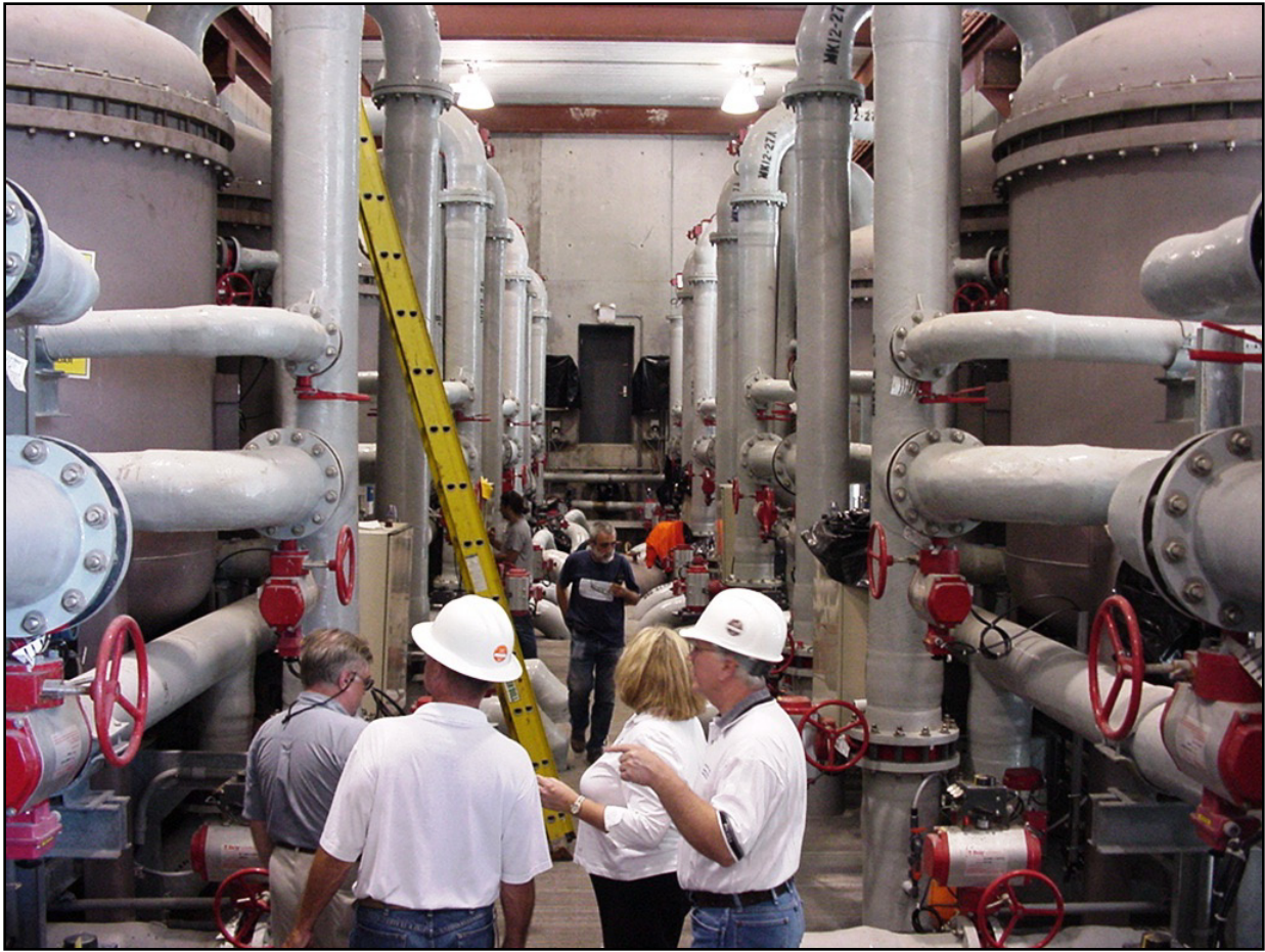
Figure D-4. Diatomaceous Earth Precoat Filter Vessels provide one of the final stages of filtration prior to reverse osmosis membranes at the Tampa Desalination Facility. (TWB, 2008)
