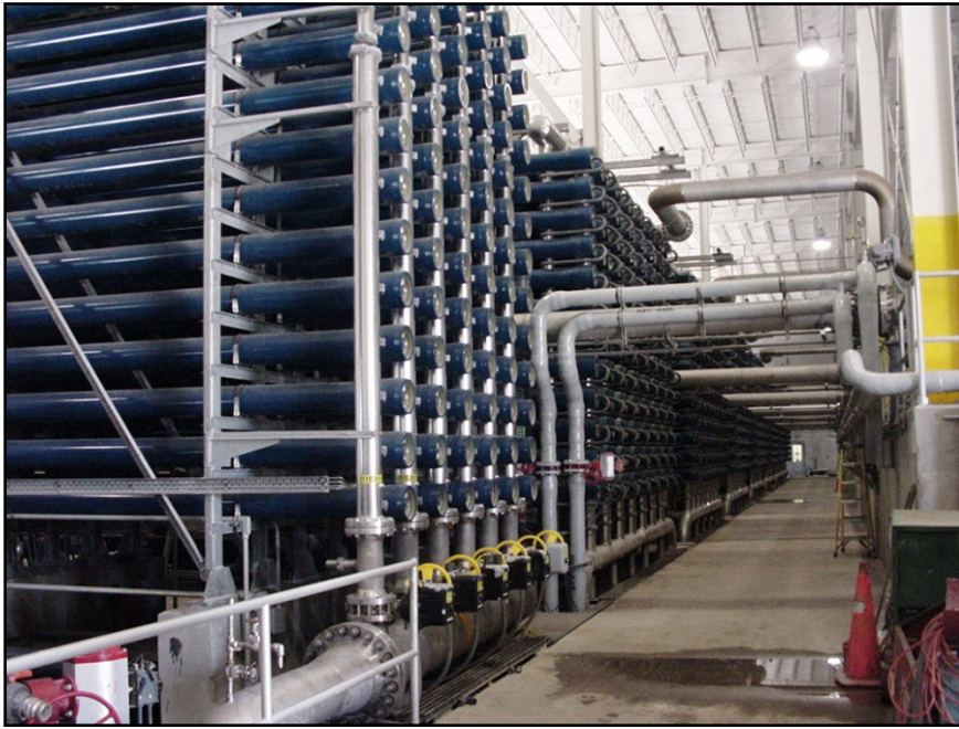
Figure 3-5. Tampa Desalination Facility Reverse Osmosis Membranes (TBW, 2008)
