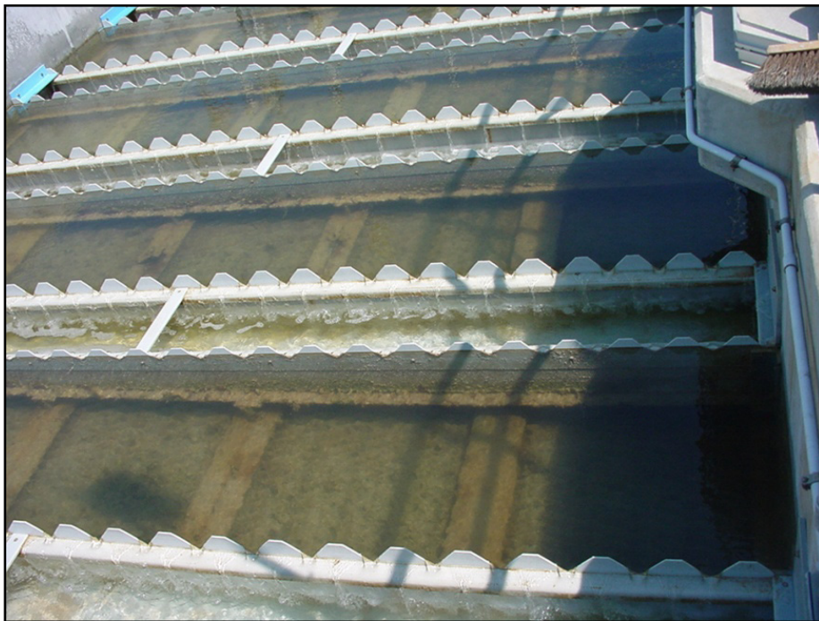
Figure D-3. Following Chemical Pretreatment the floc and sediment are separated from the water with plate settlers. (TBW, 2008)
