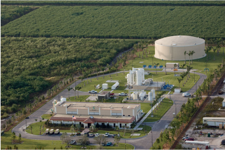
Figure 1-1. Lake Region Water Treatment Plant, Belle Glade, Florida (SFWMD, 2009)
