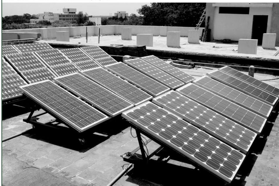
FIGURE 4 Solar Panel Rooftop System
