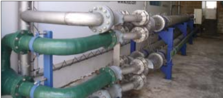
Figure 4. The eventual design comprised two identical DT250 units running in parallel.
