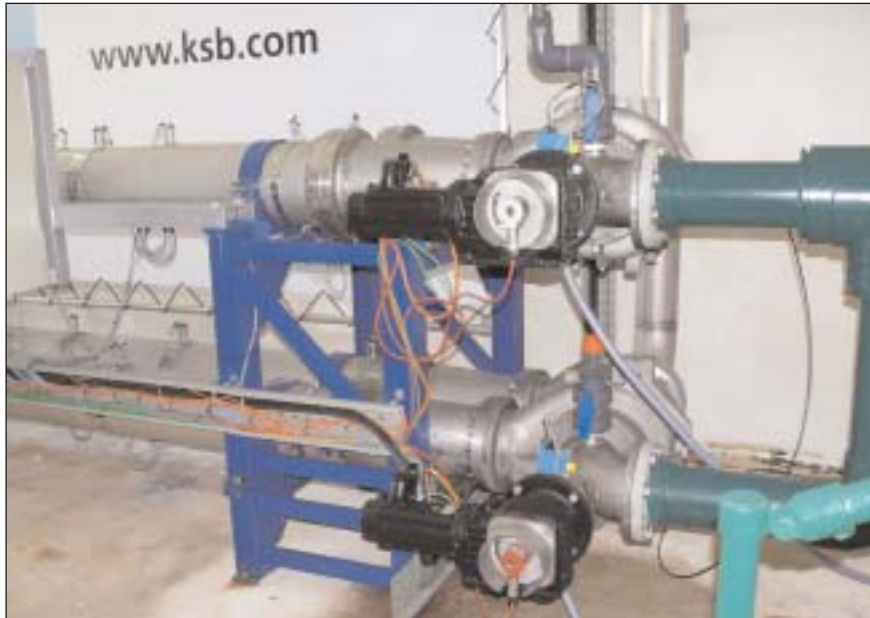
Figure 2. At the heart of the SalTec DT system is a pressure exchanger with an electronically controlled rotating valve.
