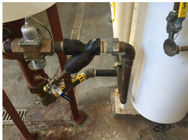
HW Skid – rear of B6, with temperature probe and 'functioning' Solenoid Valve
