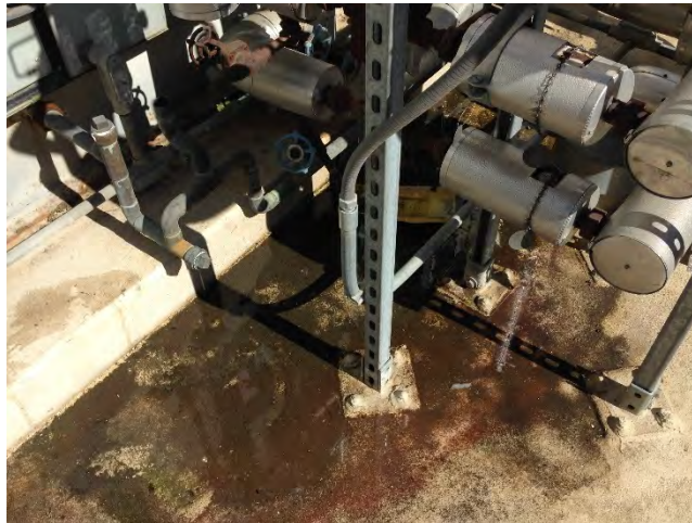
Leaking Steam Trap (Humidification) – leaking condensate on roof
