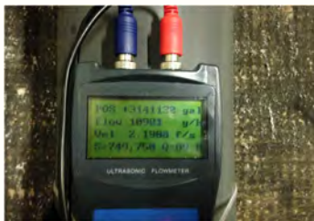
B32 Main City Water that Feeds 4 RO Trains
