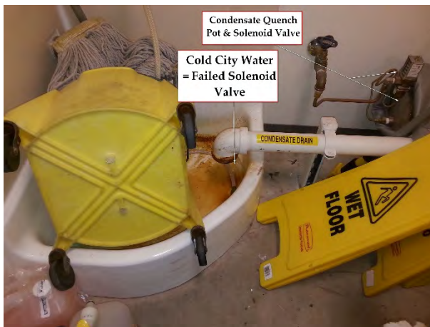
1 st Floor Janitor's Closet – Failed Solenoid on HEX Quench Line
