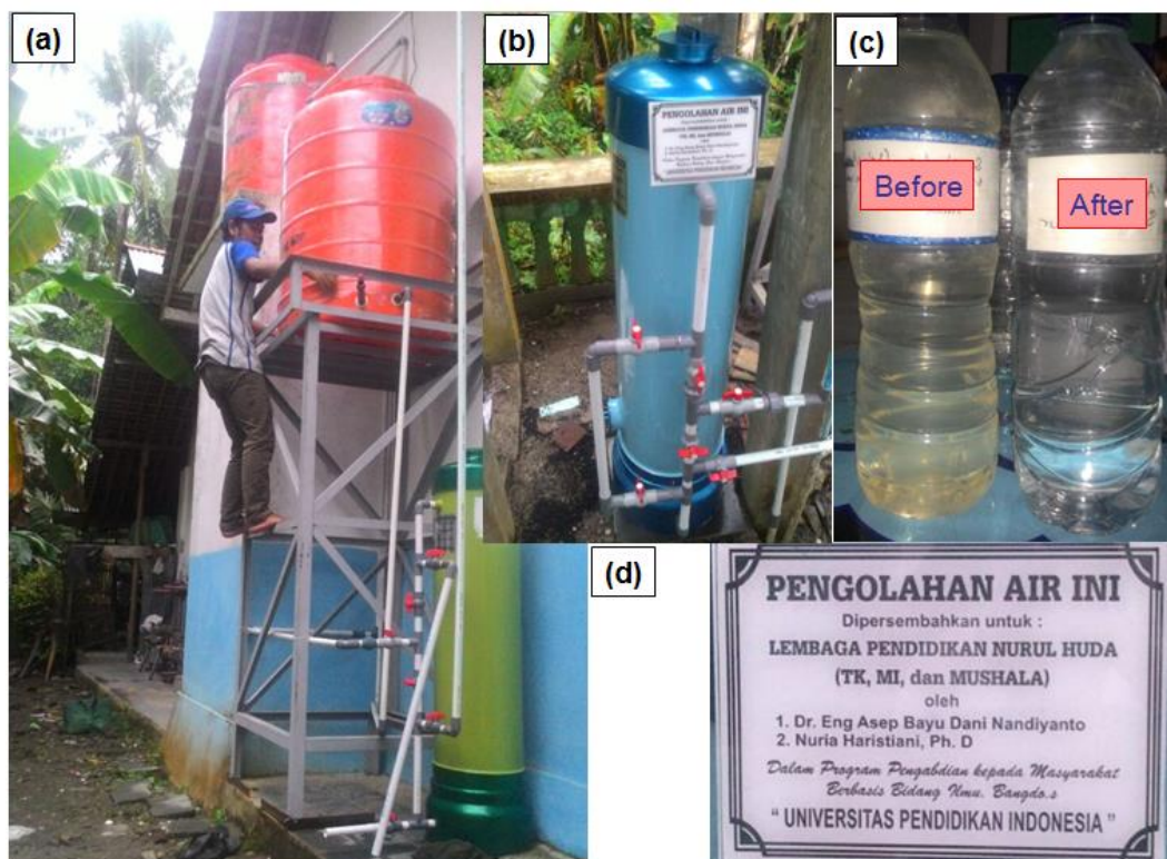
Figure 3. Appearance of water treatment system. Figure (a) is photograph image of total water treatment system. Figure (b) is the photograph image of the filter system. Figure (c) is the samples before and after the purification method. Figure (d) is the photograph image of the information regarding the fund
