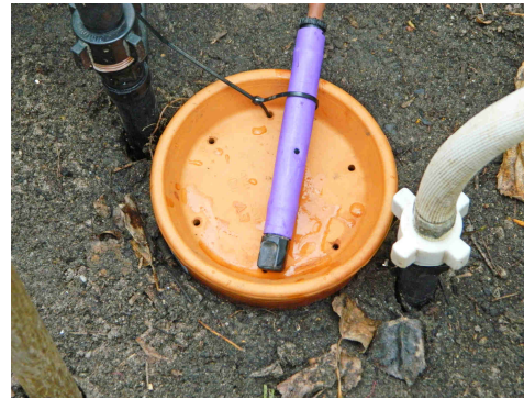
The adjustable control dripper has been replaced by an in-line irrigation dripper.
