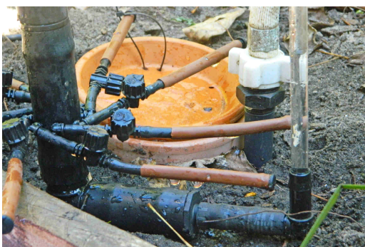
Fraction 2/7 for 8mm Netafim dripline (1 closed lower dripper, 7 open lower drippers and 2 open lower drippers as control dripper) water supply pressure 100 kPa. This setup is used for a garden in Adelaide with more than 400 drippers.
