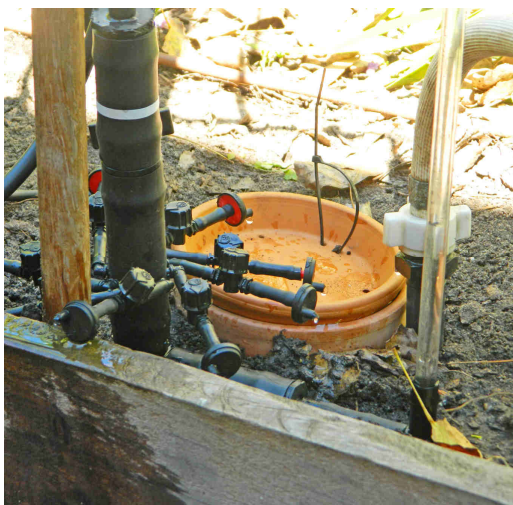
Fraction 1/8 for online drippers (8 open lower drippers, one lower dripper as control dripper) water supply pressure 40 kPa
