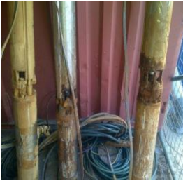
Photo 2: Pumps from various boreholes, ATW, 2014
