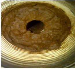
Photo 4: 80mm riser pipe from W34012, Witzands, 2014
