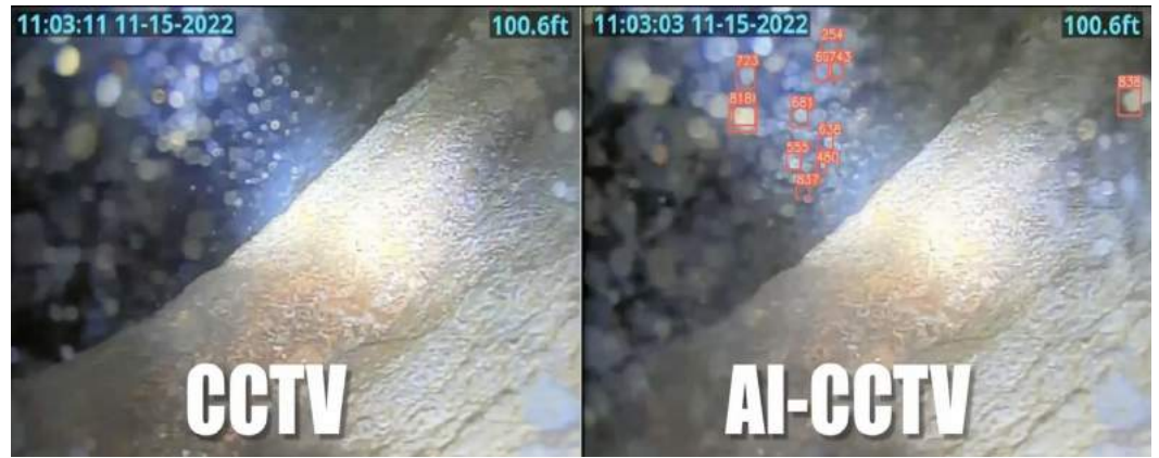
Figure 39. Electro Scan AI Uses High Resolution Cameras to Track and Confirm Leaks Found in Pipes.
