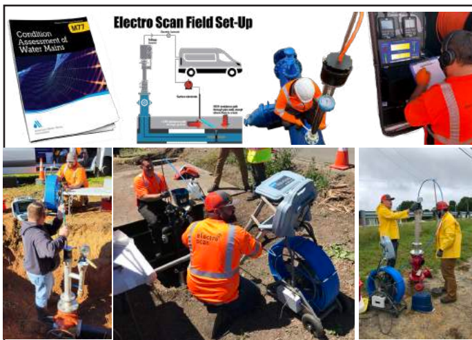
Figure 36. Example Electro Scan Pressurized Pipe Insertions into Live Drinking Water Pipes in Accordance with AWWA M77 Standard (2019).
