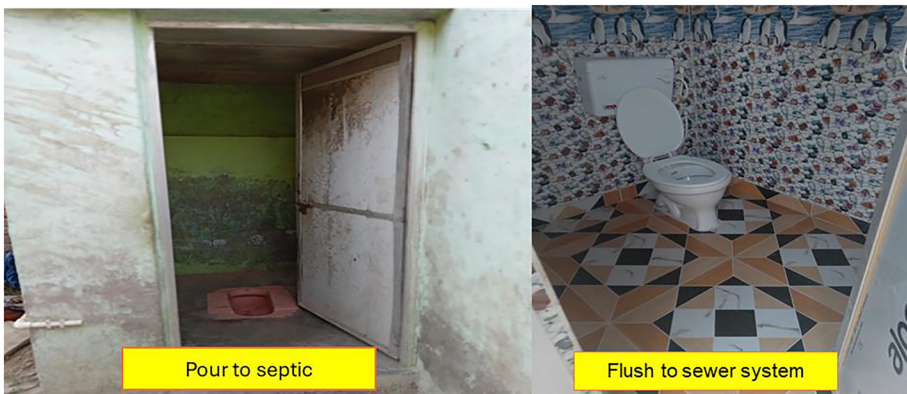
FIGURE 7 Two types of toilet facilities used in the village.
