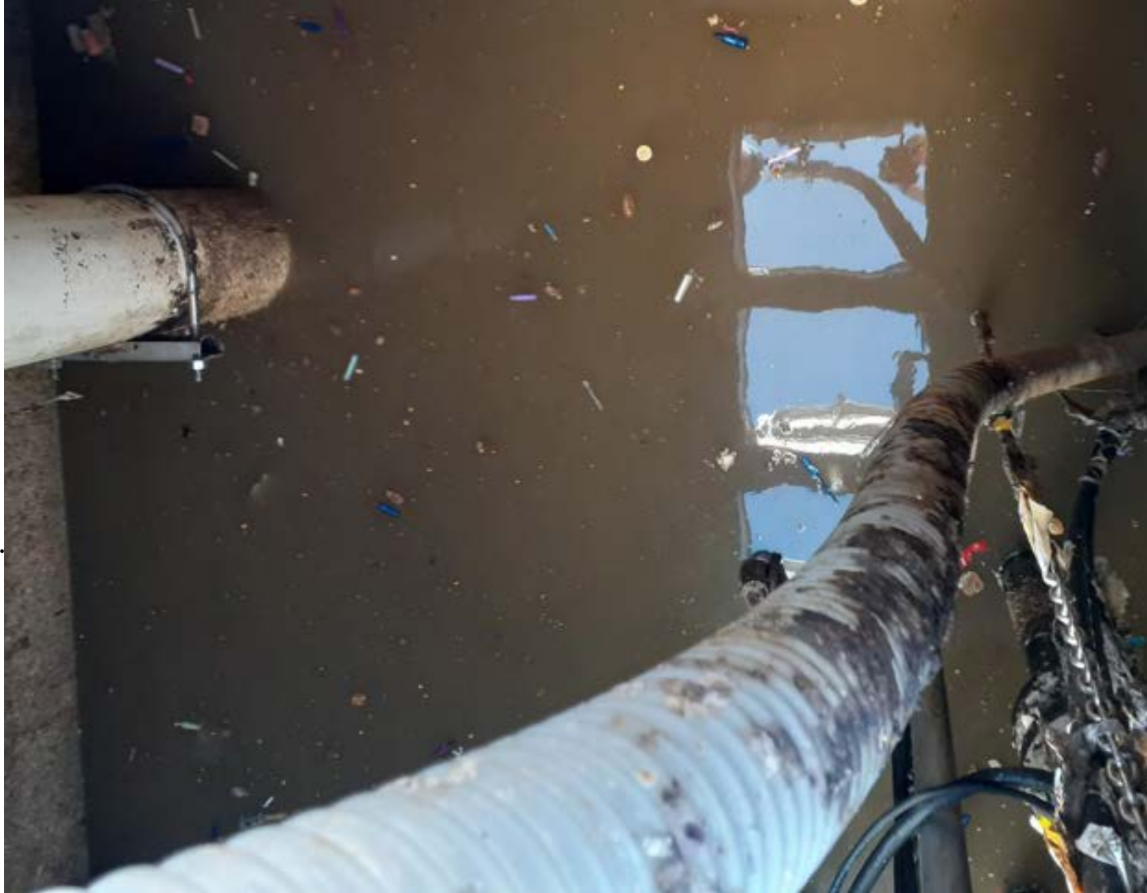
There used to be a seven feet thick layer of grease at Lift Station #8, but not any more.
