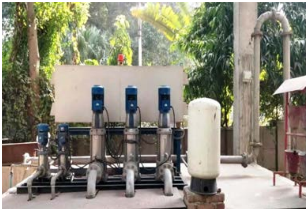
Pumping Station at West End, Delhi
