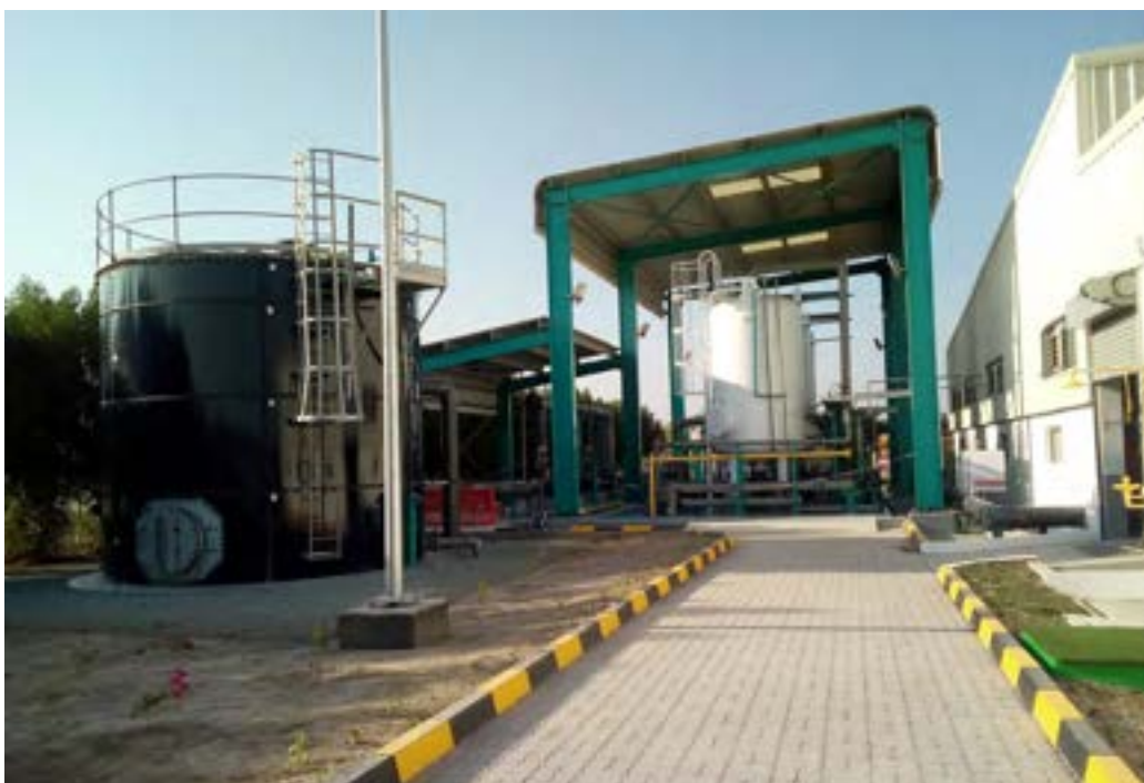
HMRU at CETRP Majis Plant in Sohar Industrial Area, Oman
