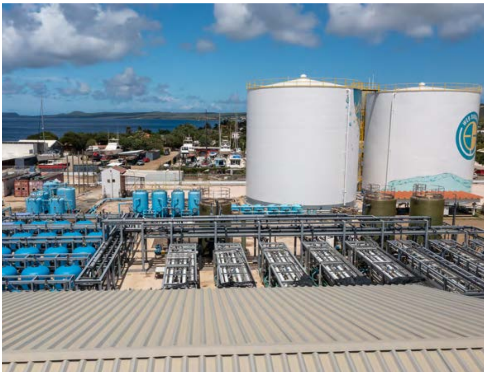
The Plant Offers a High Level of Preassembly of Sub-systems, Allowing Efficiency in Construction and Providing Extremely Low Electrical Consumption.
