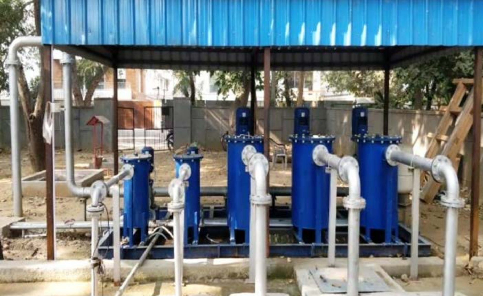
Pumping Station at Shanti Niketan, Delhi
