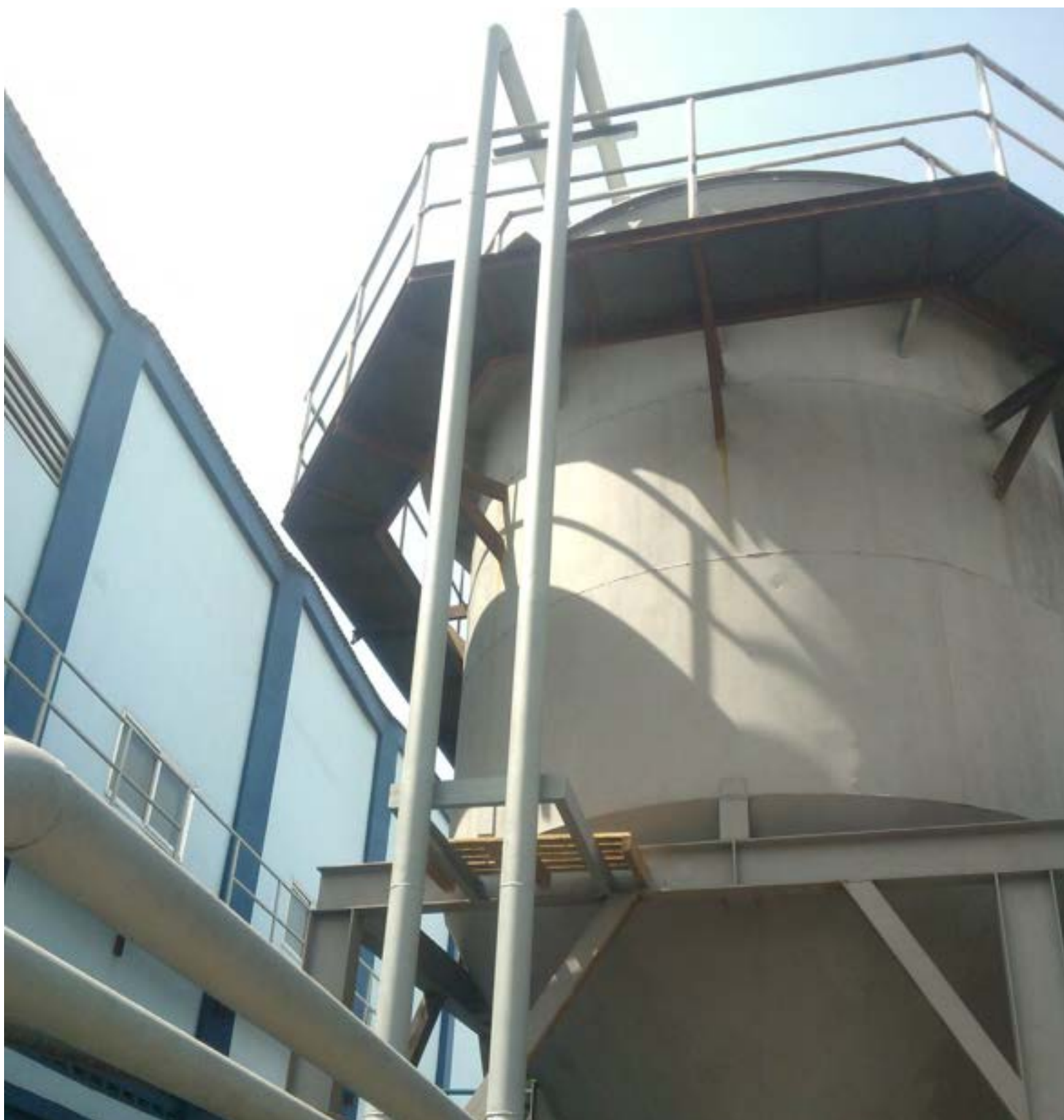
Inlet Pipes to the Clarifier
