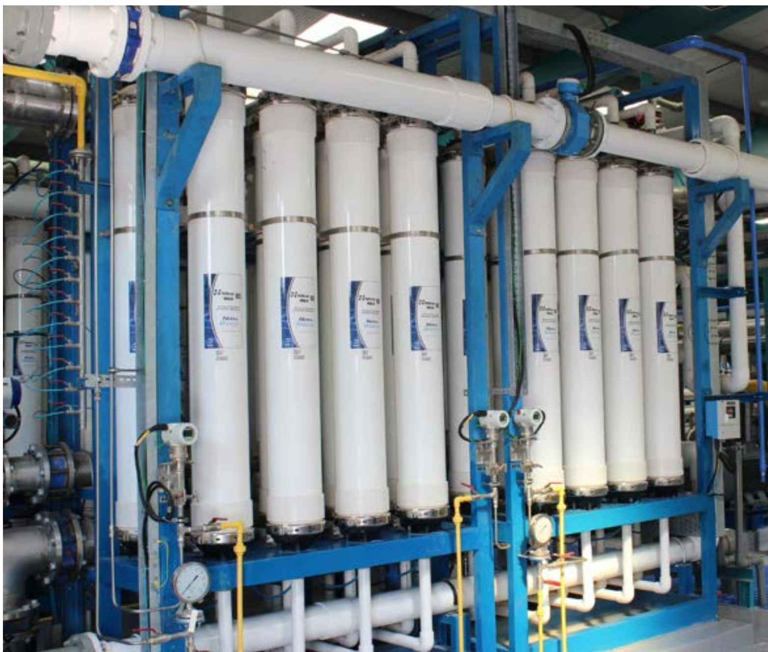
UF rack inside CETRP Majis Plant in Sohar Industrial Area, Oman
