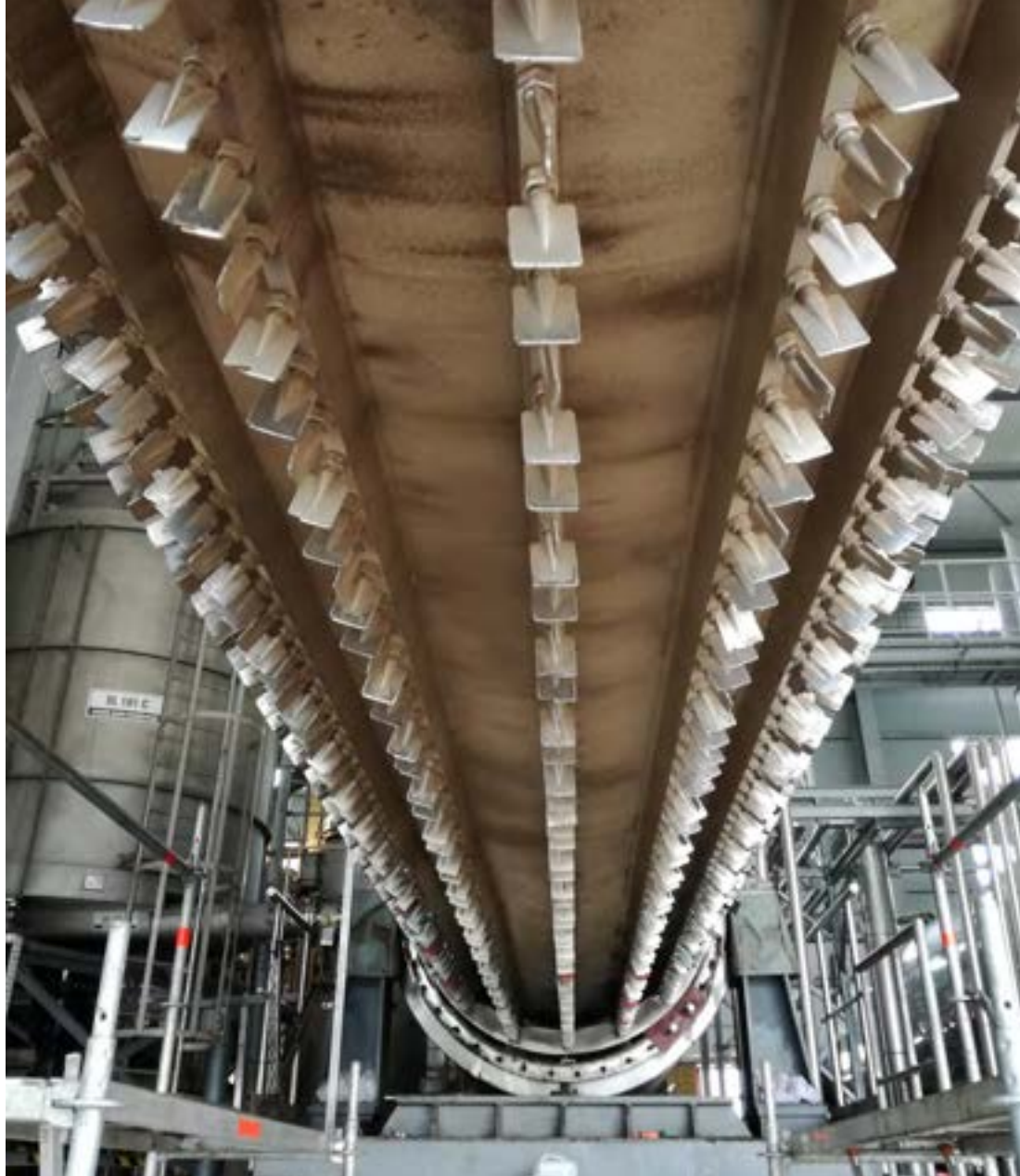
The mechanics of the drying rotor are very complex. Shown here during inspection, this equipment needs to be adjusted carefully to avoid damage and optimize performance.
