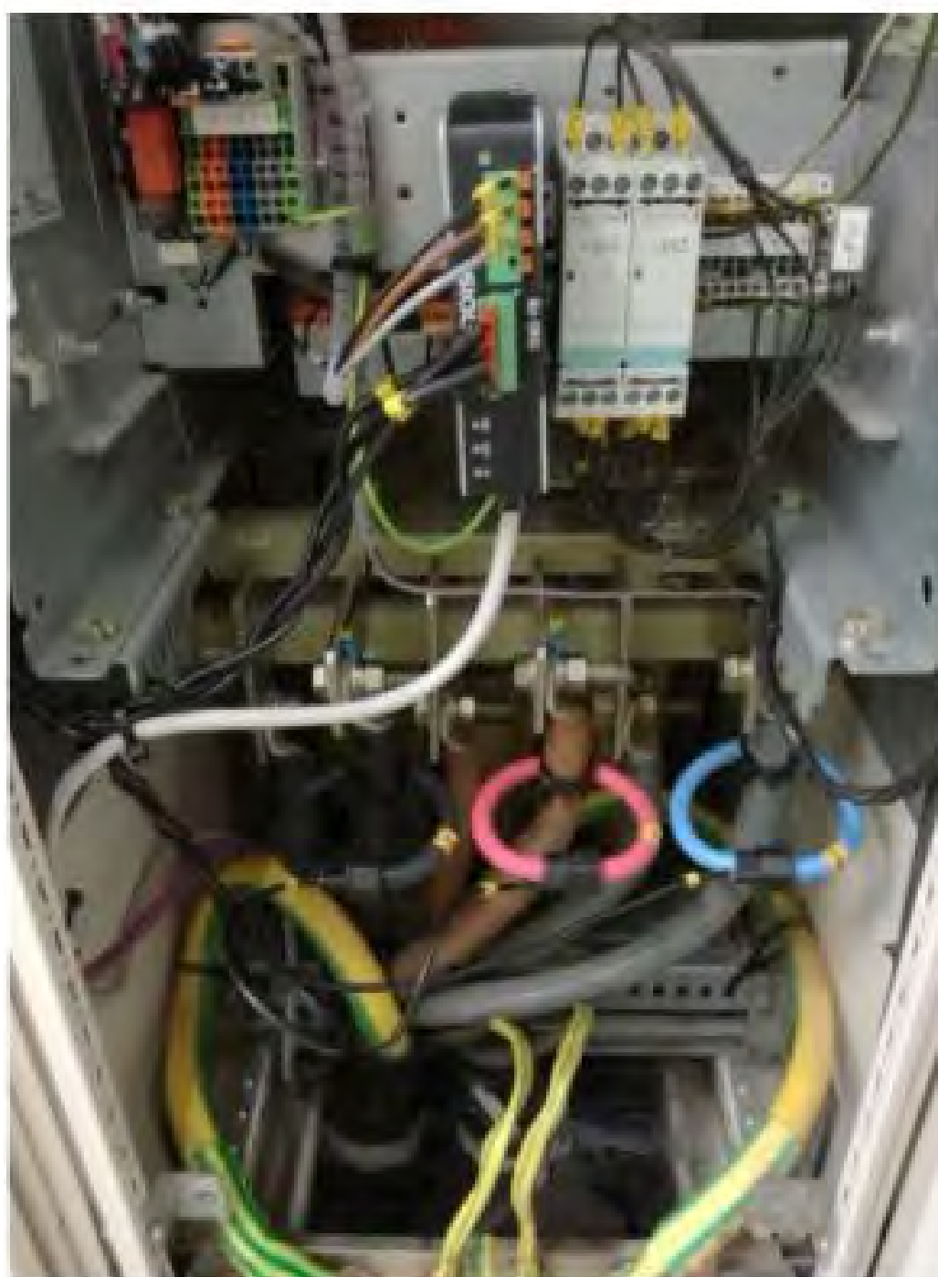
The Elmodis sensors and controllers were installed throughout the system, such as in this inverter cabinet, to measure more than 500 parameters involved in the dryer system operation.
