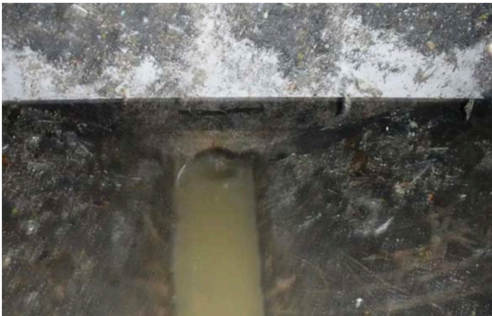
Reduced flow due to sewer blockage in Bath catchment
