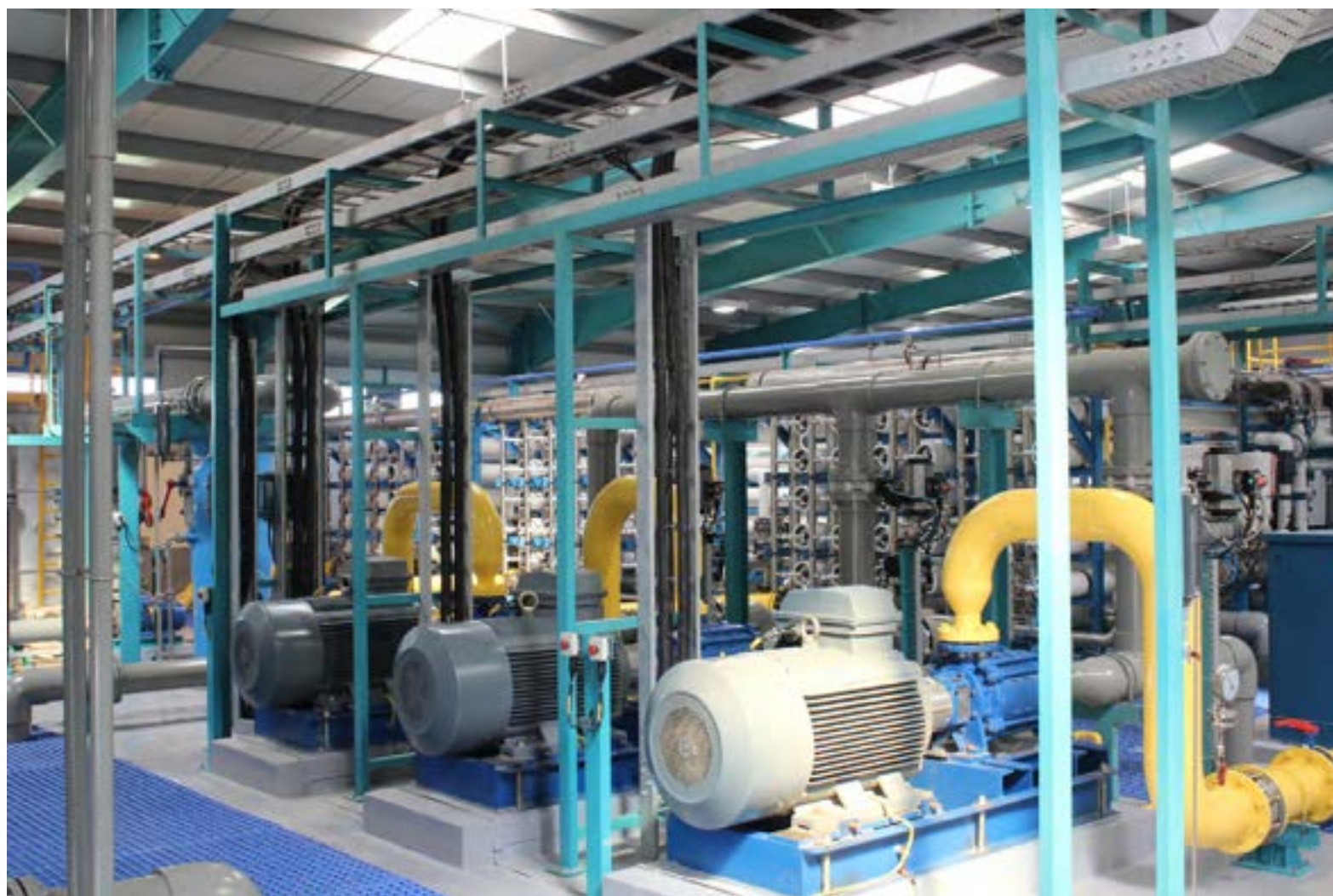
RO section inside the CETRP Majis Plant in Sohar Industrial Area, Oman
