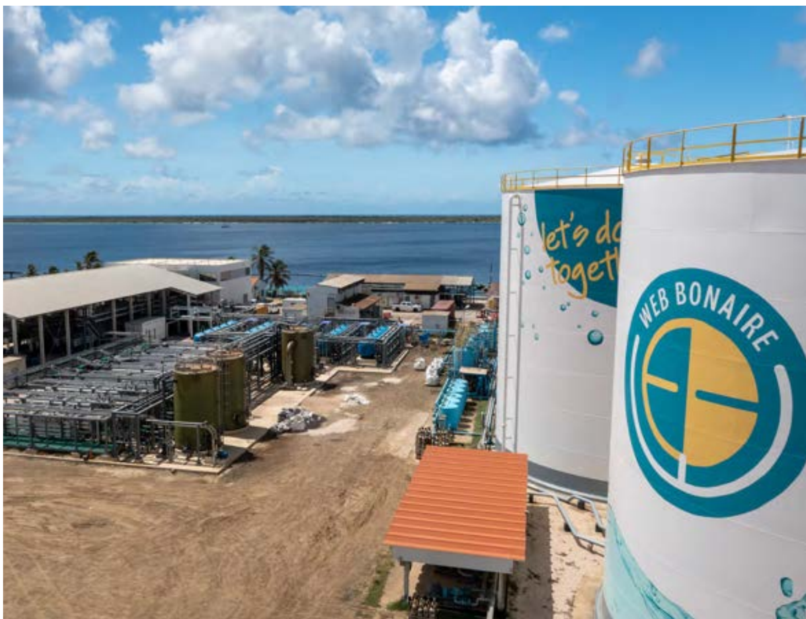
Bonaire's New Plant Produces 5,600 m 3 /d of Drinking Water to Meet the High Demands of the Island's Nearly 22,500 Residents.
