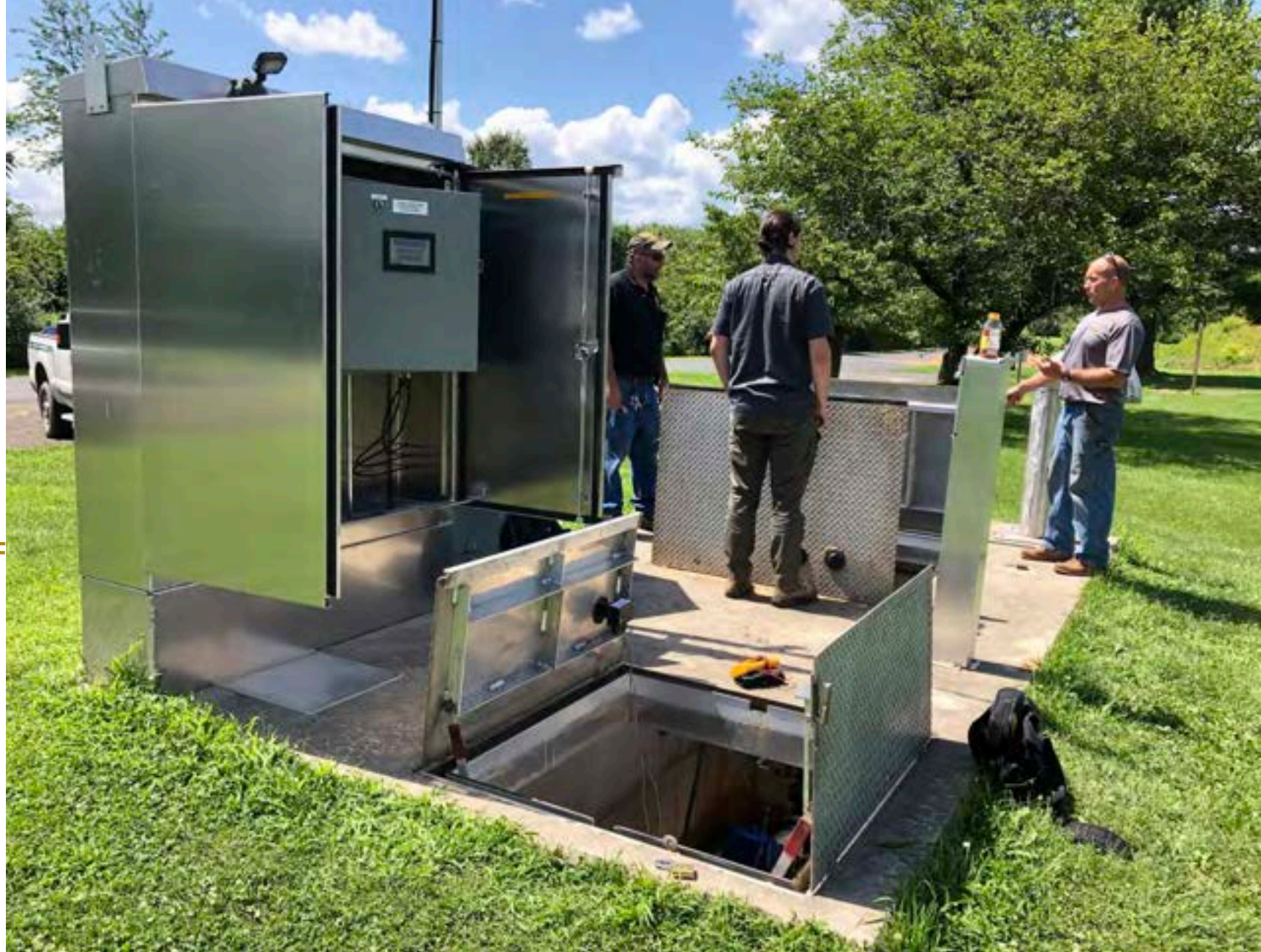
Mueller works side by side with their partners and end-users to commission the system and train operators how to make most efficient use of the technology.
