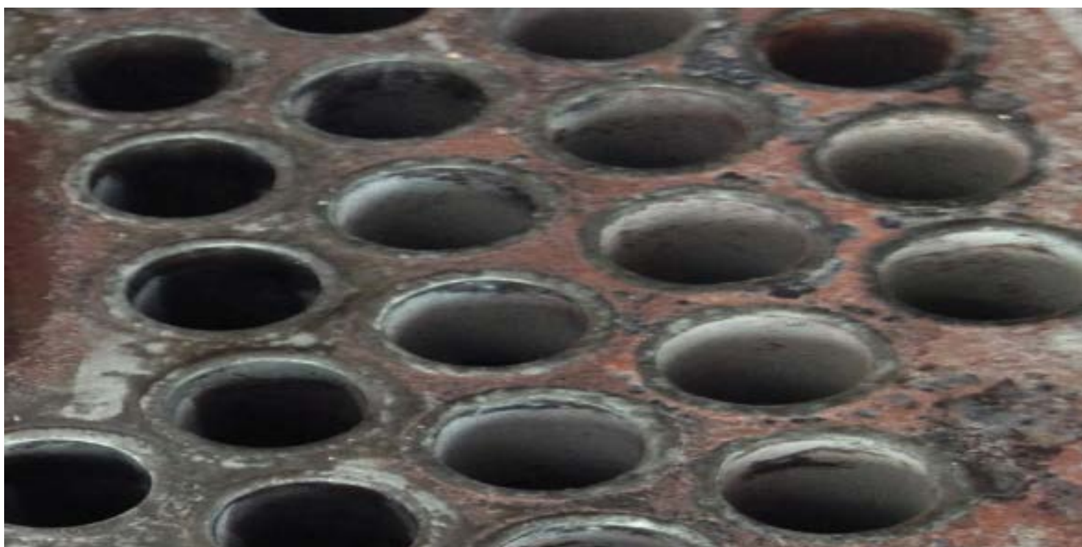
Formation of deposits without Activepowerclean
