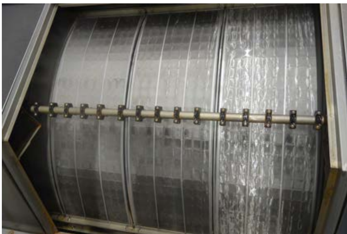
45 filter panels with the high-performance Porometric mesh from GKD with the required pore size of 25 µm are used in the drum filters at Swiss Alpine Fish.
