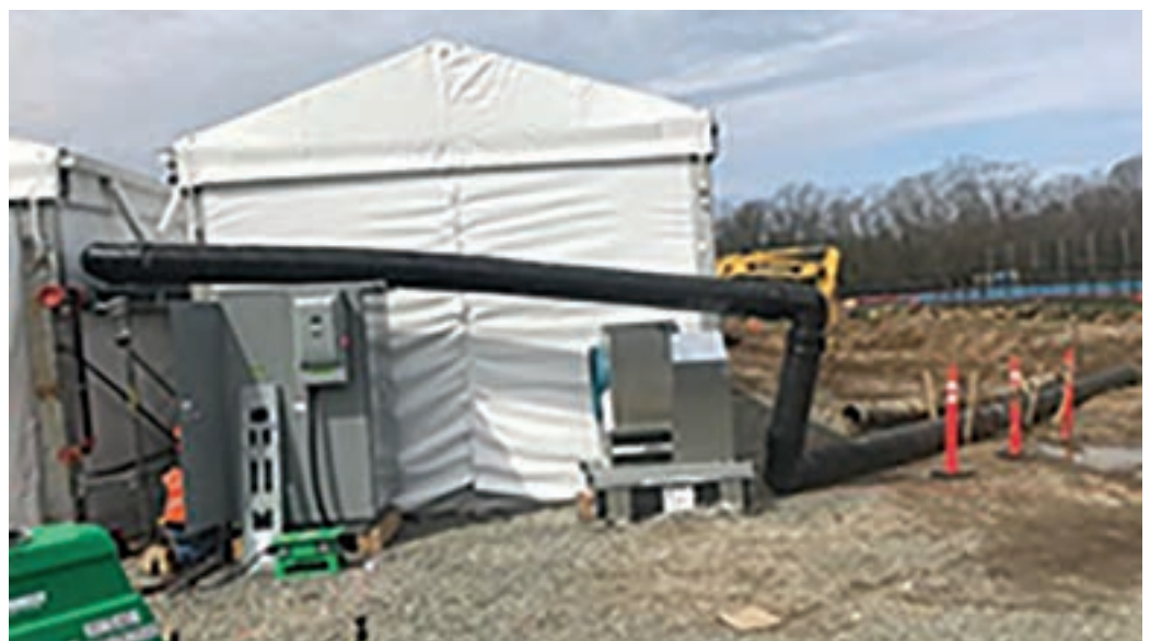
ADS N-12 pipe was used to convey rain water from the roofs of the field hospitals at Stony Brook and SUNY Old Westbury, New York.
