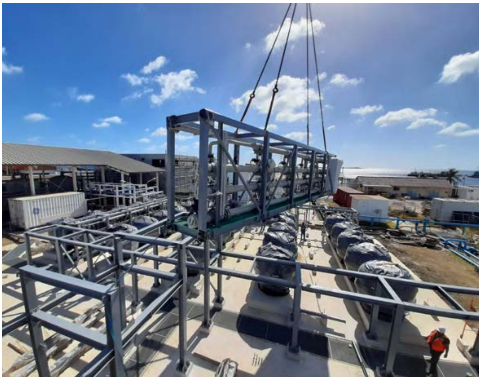
Through WEB Bonaire and IDE's Partnership, They were Able to Design and Build the Facility Under COVID-19 Constraints and Complete the Entire Facility Within a Year and a Half.
