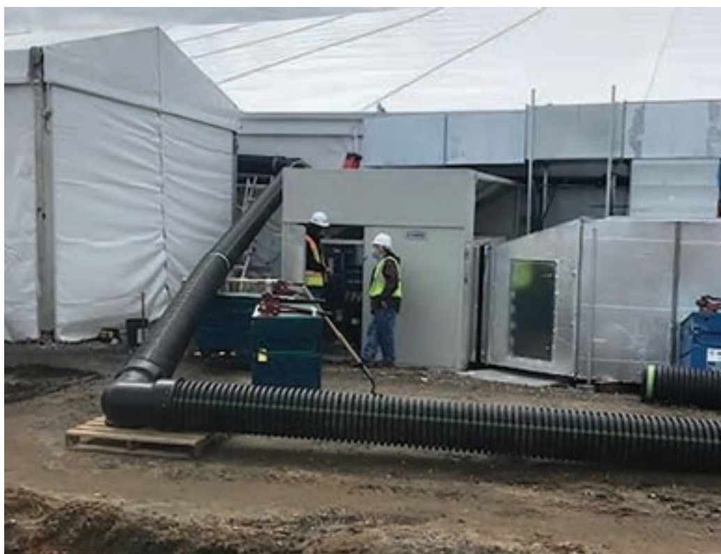
Rain water is conveyed from the roof to gutters then to ADS N-12 pipe where it drains into swells.
