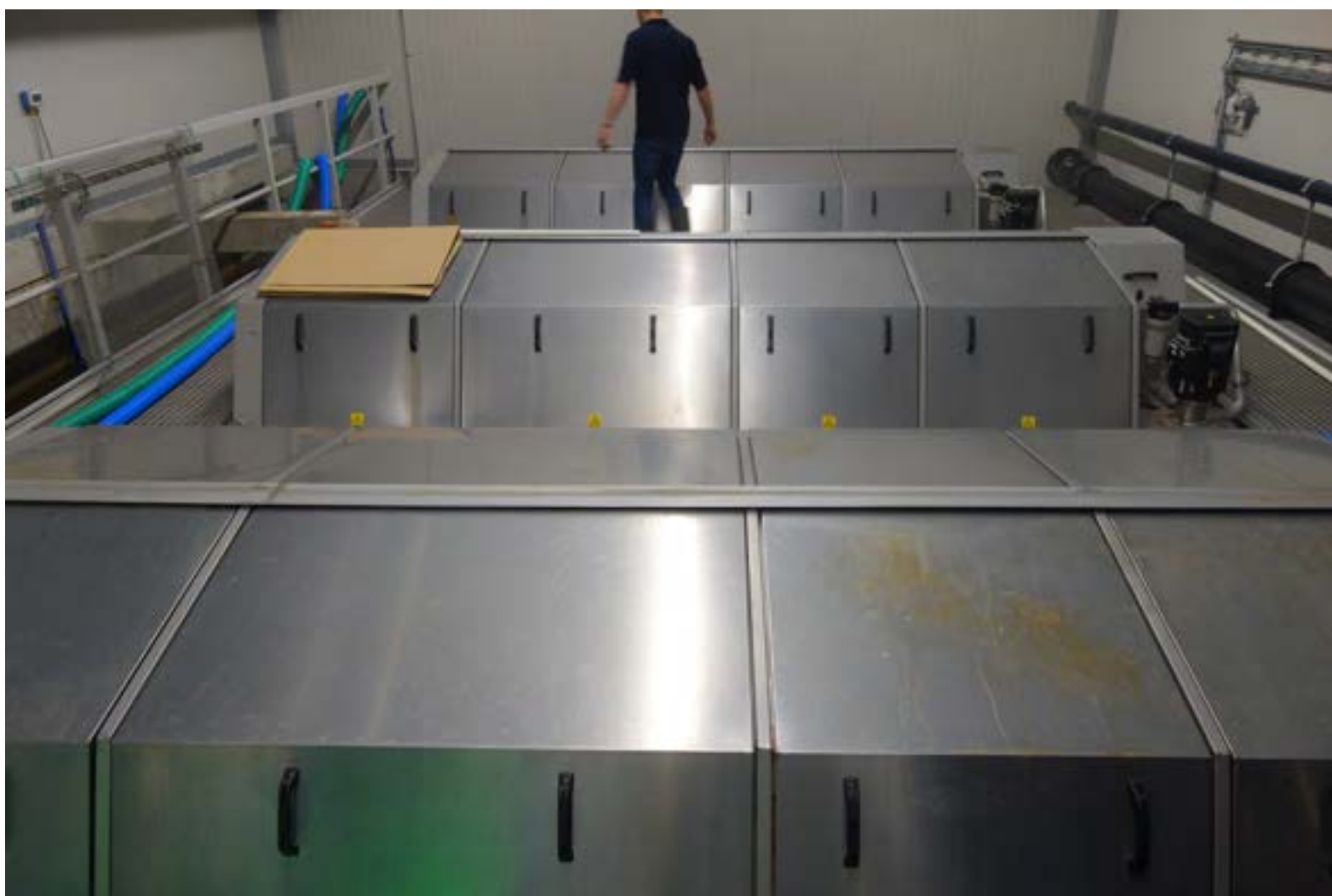
Three HDF 2009-1AS drums filters are used at Swiss Alpine Fish to clean the water mechanically.
