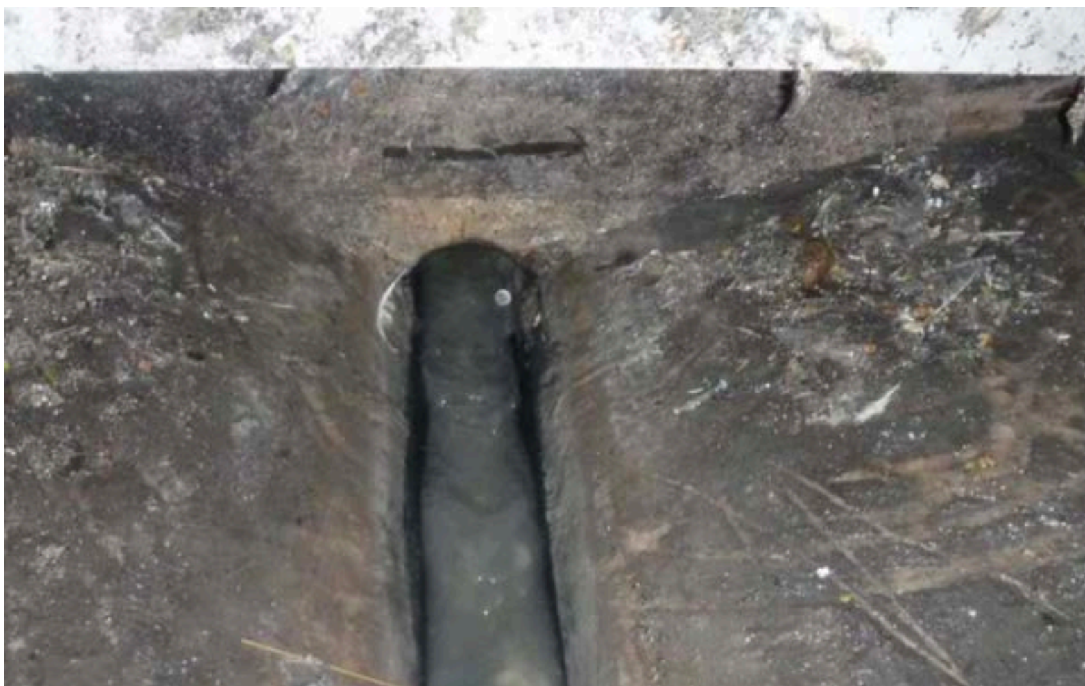
Unrestricted sewer flow in Bath catchment
