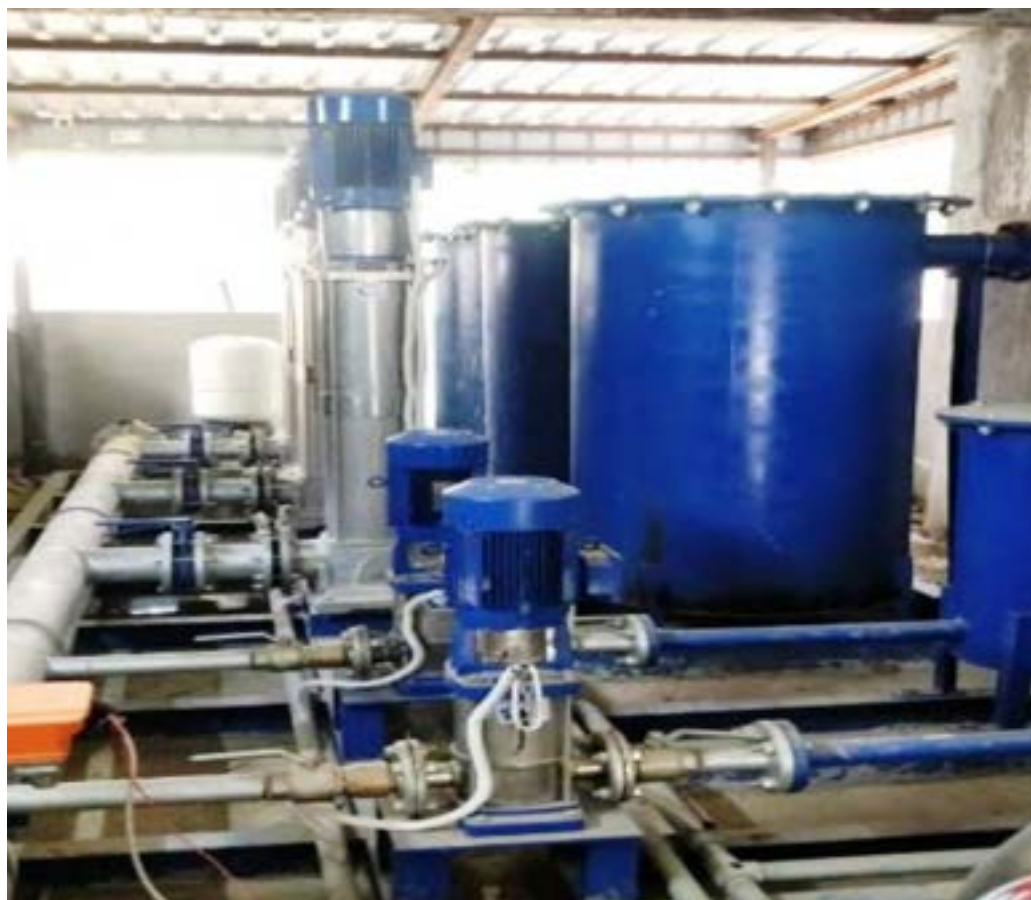
Pumping Station at Anand Niketan, Delhi
