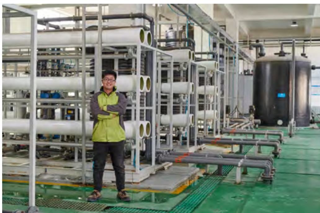
The deep membrane treatment facility for leachate water at the Daxing landfill for Shenyang, with Operations Manager Zhang Shuai of WELLE.
