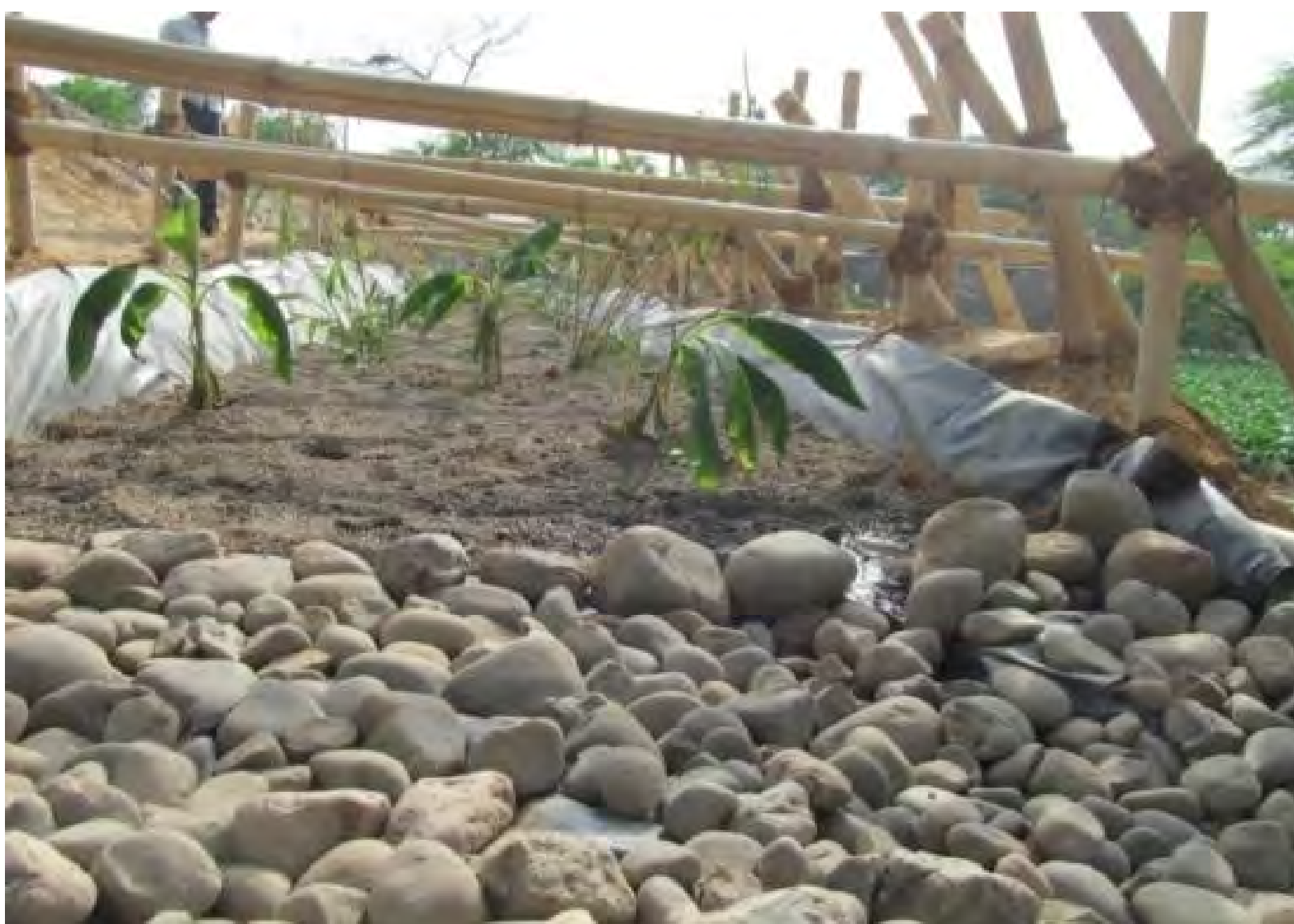
Constructed Wetland to Treat Wastewater from a Slum in Delhi
