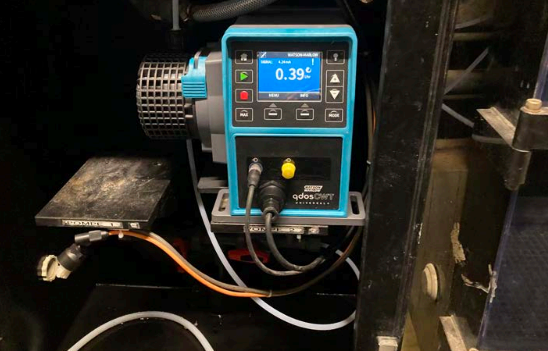
Qdos CWT Installed at Villejean Water Treatment Works
