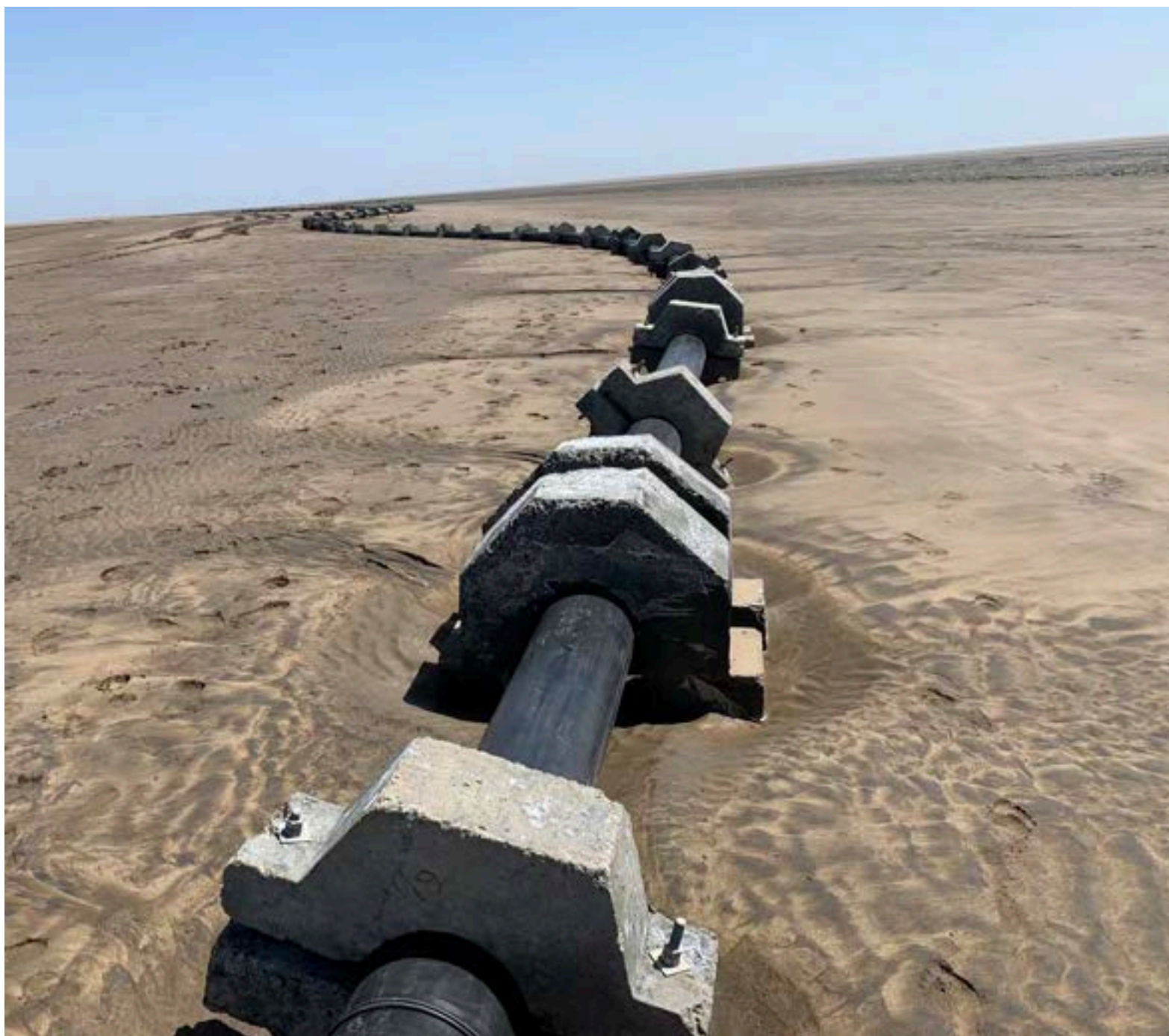
HDPE pipeline weighed down by concrete sinker blocks in the inter-tidal zone
