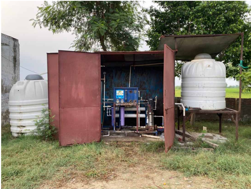
Fig. 3 | Water treatment plant at Nagla Chandi (Jivamritam).
