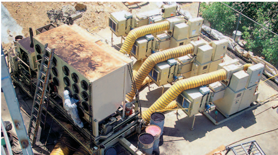
Polygon desiccant dehumidifiers held-the-blast and saved more than $4,000 per week in a Southern California water tank coating job. A four million gallon municipal storage tank was blasted and re-coated, while a white metal blast was held for over three weeks.
