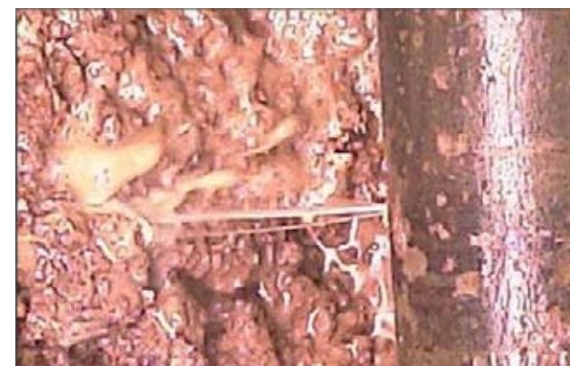
Figure 10 Leak found by Zonescan
