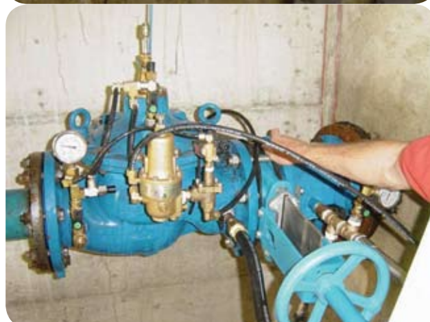
Photos of the flow modulation PRV having a hydraulic control
