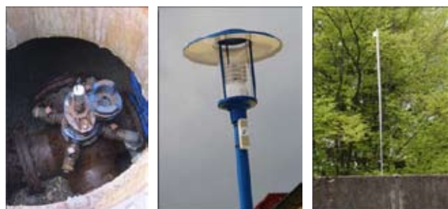
Figure 6 – Installation pictures of the noise logger, radio repeater and GPRS data collection unit left: Zonescan Correlating noise logger deployed magnetically on a hydrant centre: Zonescan Repeater installed on Streetlamp right: Zonescan Alpha installed on a mast above the water tower
