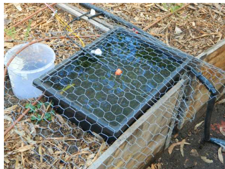
Evaporator, float switch and control dripper for zone 2
