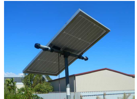
Solar panel mounted on a pole
