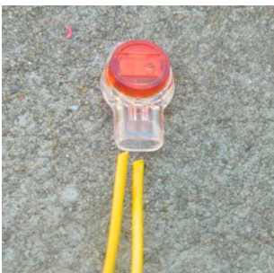
Wires are not stripped before insertion
