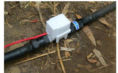
Solenoid valve installed at ground level
