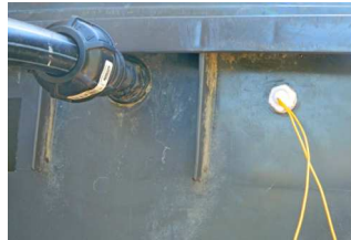
Float switch on the header tank is lower than the inlet
