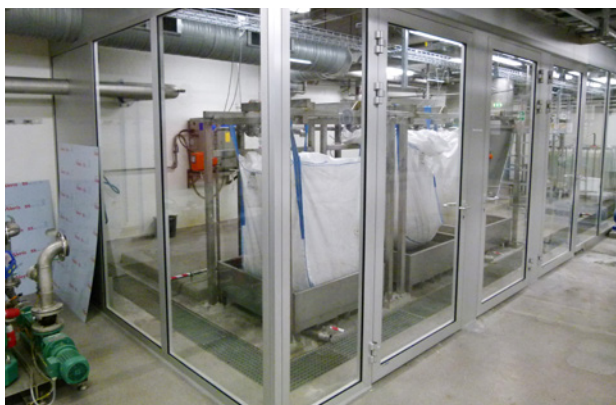
Struvia™ installation in shielded area in basement
