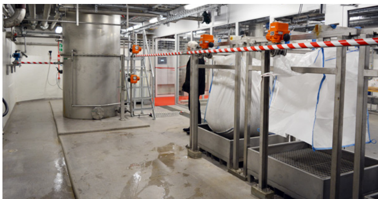
Struvia™ reactor and struvite drainage system
