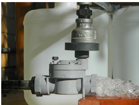
When the magnet is in the low position, the magnet lifts the plunger inside the solenoid and opens the valve
