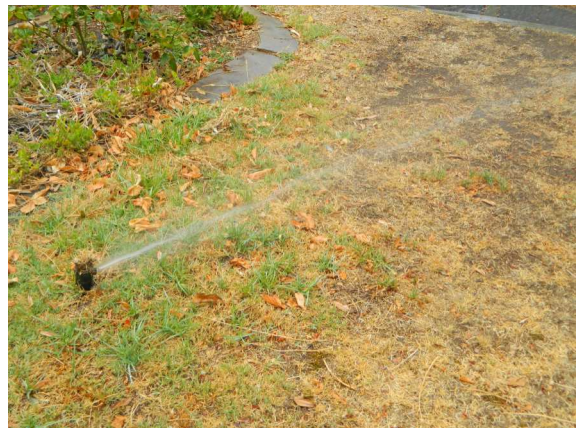
The solenoid valve opens and the irrigation starts
