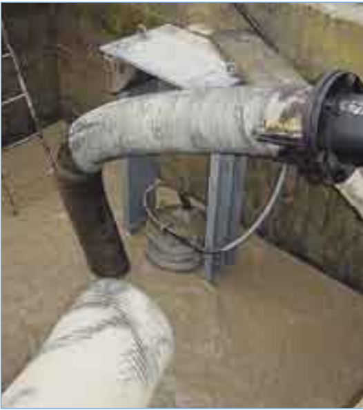
THY35B: reflux water pumping in the marble cutting industry (Italy).
