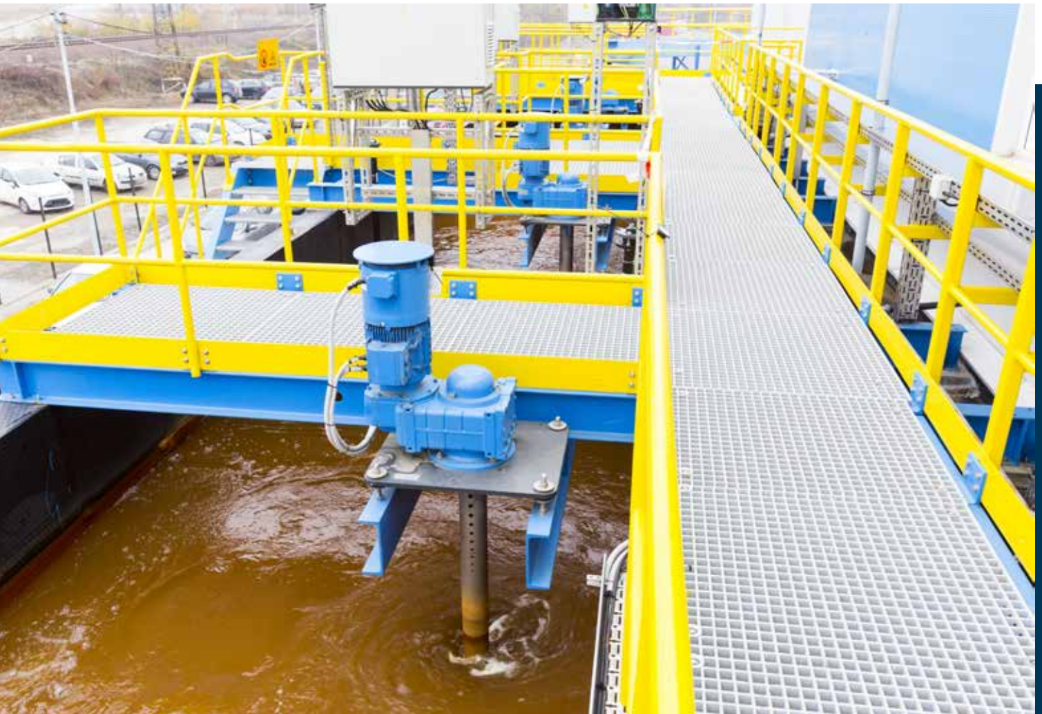
Rainwater treatment plant Photo: © Cylonphoto/Shutterstock.com
