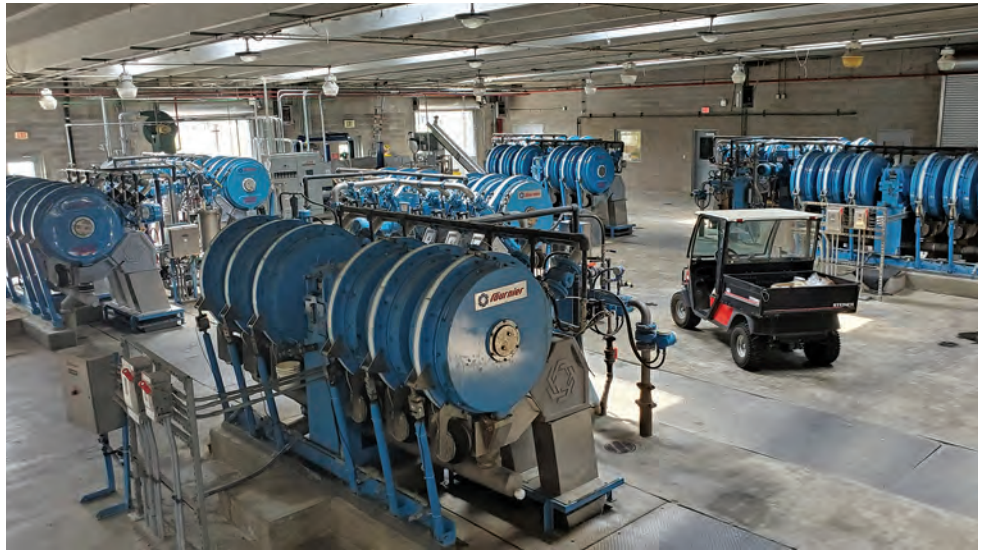
The biosolids produced at the high-performance Murfreesboro facility are dewatered on eight rotating sludge presses (Fournier Industries) and are currently being landfilled.
