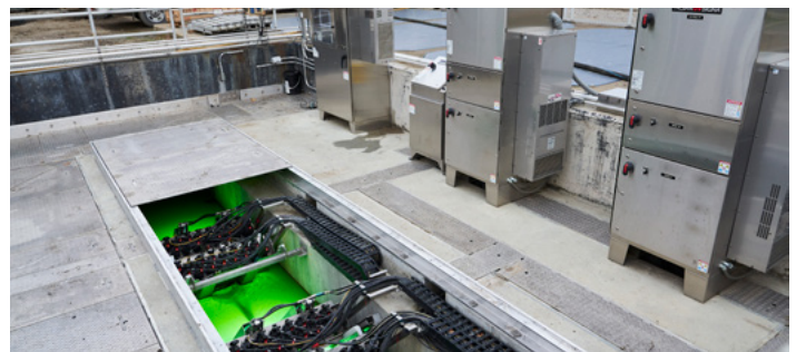
This TrojanUVSigna installation can treat 20 MGD (875 l/s) in only 250 ft 2 (23 m 2 ).
