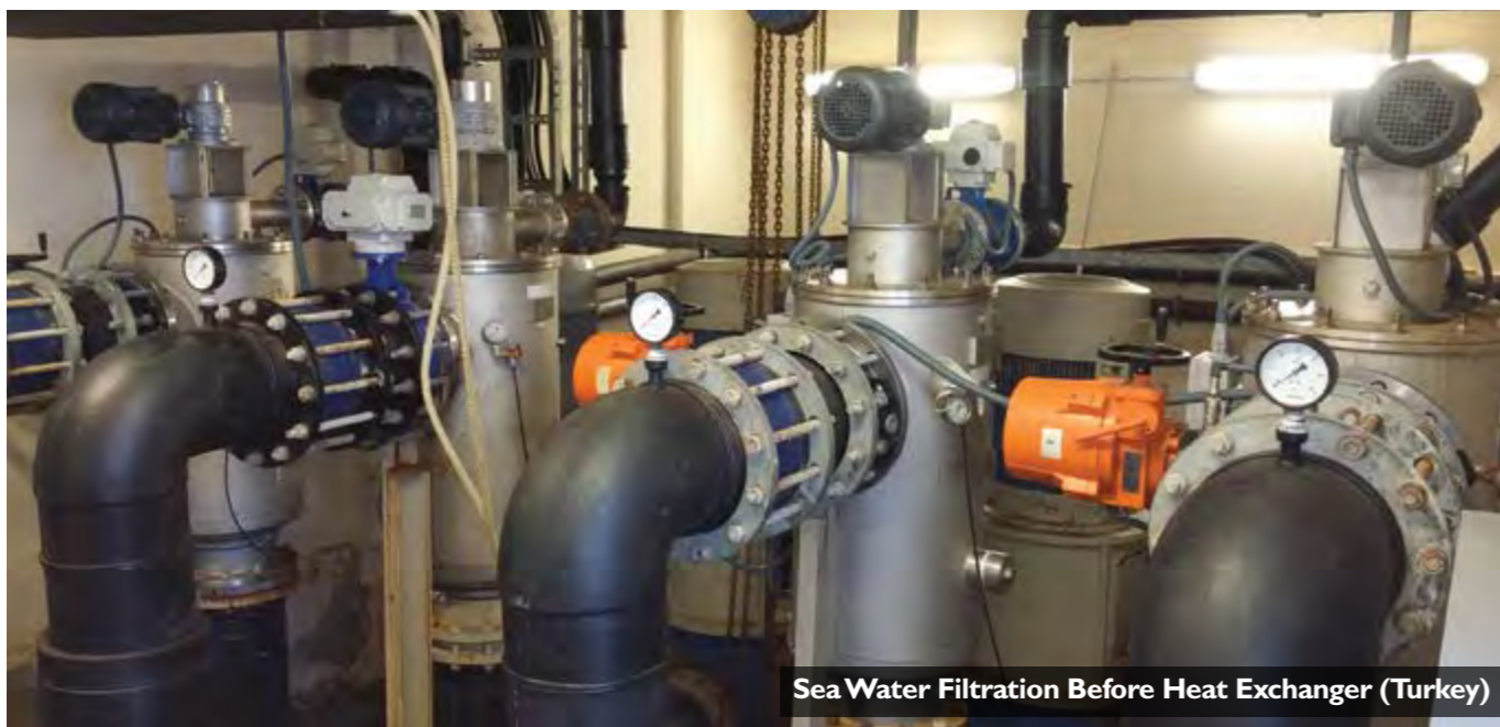
Two Stage Filtration of Sea Water Before RO and Desalination (Kingdom of Saudi Arabia)
