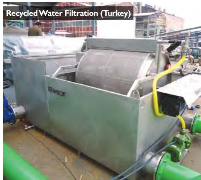
Treated Waste Water Filtration Before UV (Turkey)
