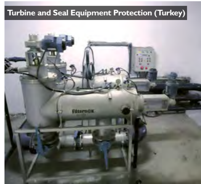
Turbine and Seal Equipment Protection (Turkey)
