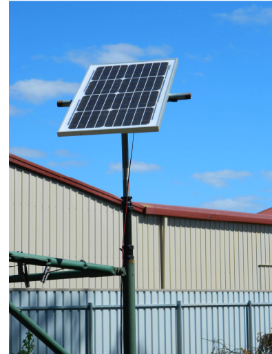
20 watt solar panel mounted on a pole
