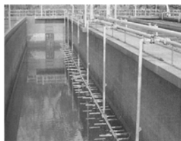
Diffusers near bottom of empty aerator
