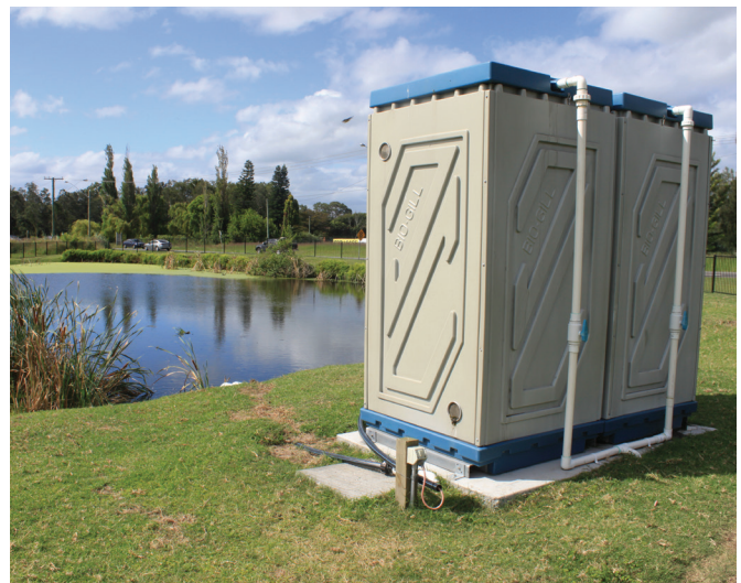
BioGill bioreactors treating wastewater onsite at Tomago.
