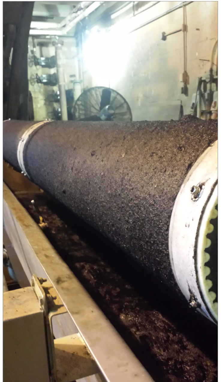
Installed System Operating at National Beef
