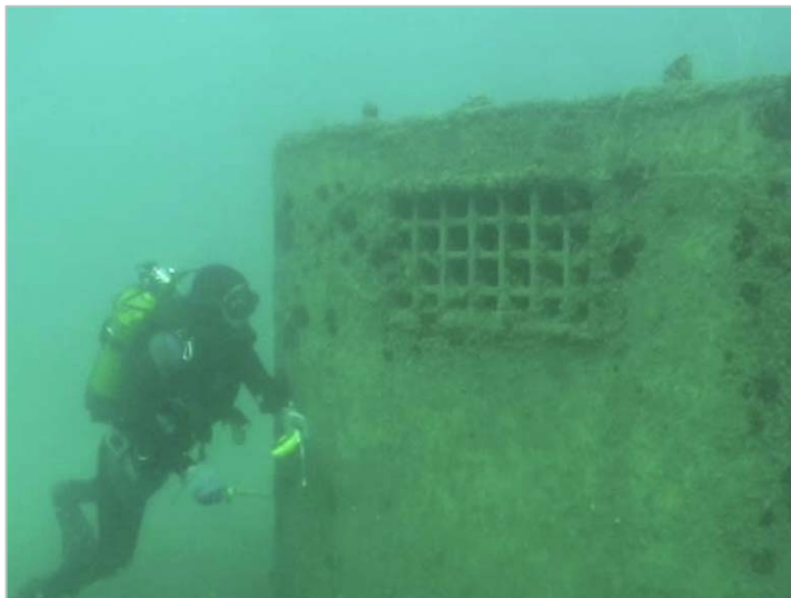
An intake with hipochlorite addition out of work
