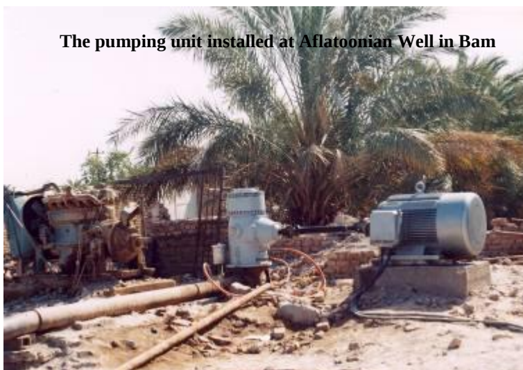
Aflatoonian Well before the new units were installed
