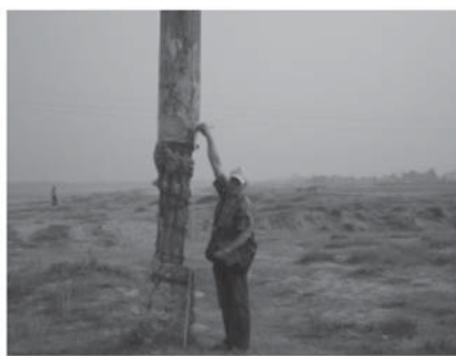
Figure 8. Electric pole hanging
