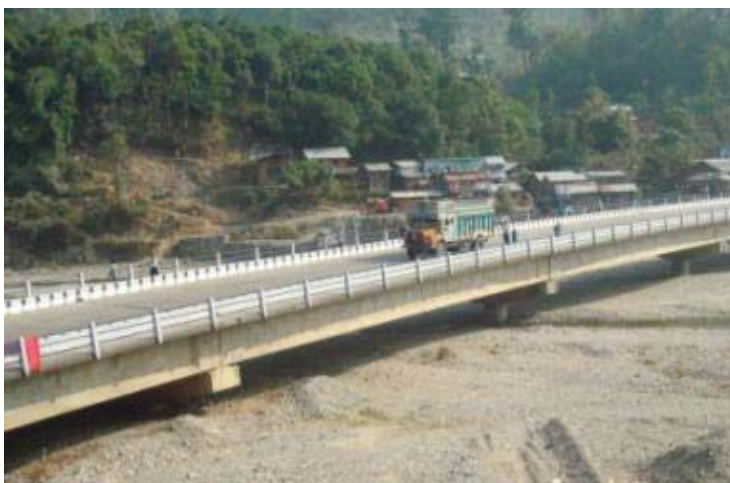
Photo 2. Sediment Accumulation under the Lothar High Bridge.
