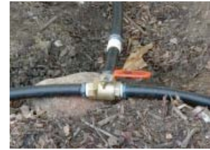
Photo above: 3-way valve to enable the alternative irrigation of 2 different zones to avoid waterlogging of an area (Note: here the system is not fed by gravity).
