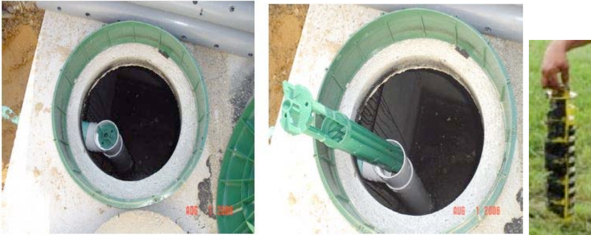
Effluent filter in place at the septic tank outlet. To clean the filter, it is simply lifted out and hosed off, with the solids falling back into the tank.
