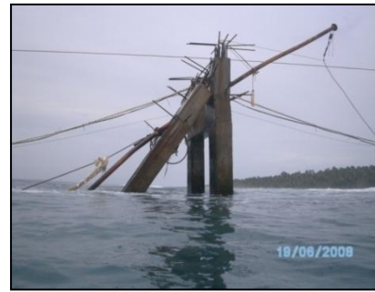
Fig. 34 Damaged pier 12 due to high waves
