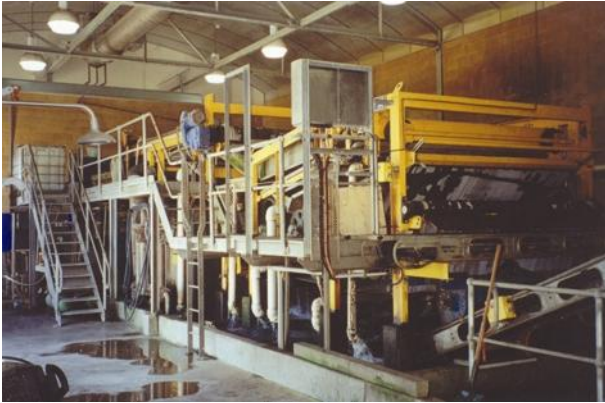
Sewage Treatment Plant (internal shot)
