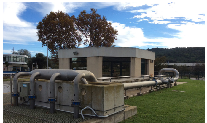
Figure 5. Castell - Platja d'Aro Water Reclamation Plant.
