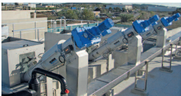
3 RPPS-Star screens size 1000 with 1.5 mm perforation protecting the downstream membrane plant
