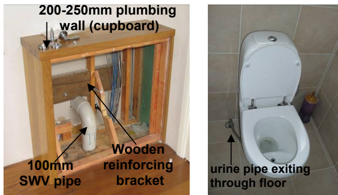
Figure 2: (a) Wall modification to fit rear plumbing (left) and (b) Gustavberg wall mounted UST with incorrectly modified urine pipe (right).
