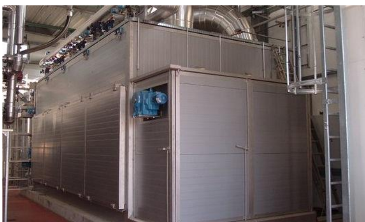
Figure 60 - Low Temperature Belt Dryer in German (Huber)
