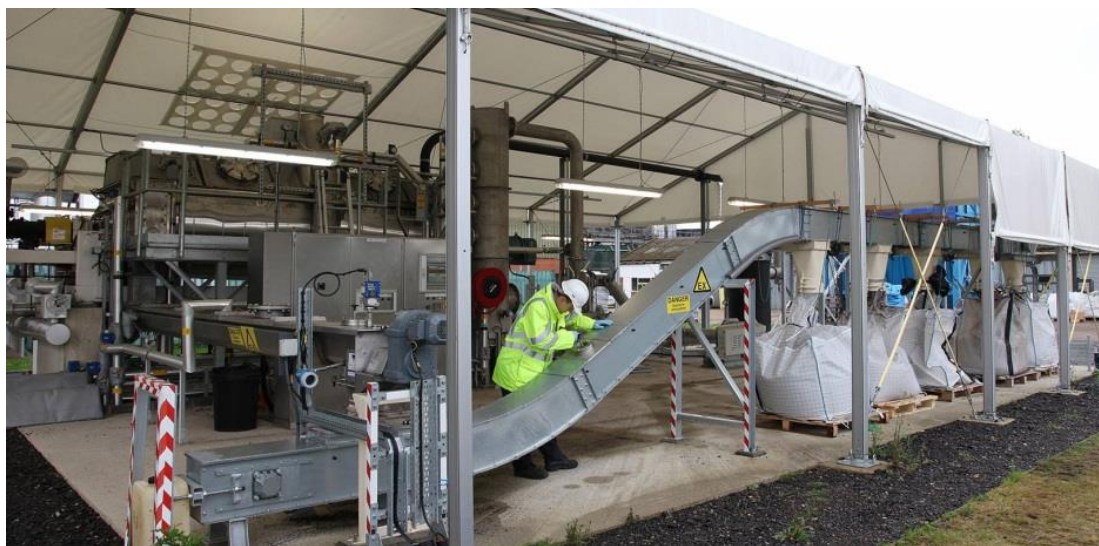
Figure 2 – The paddle dryer demonstration plant at Slough (4.5 Tonnes / day)
