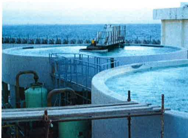
Dissolved air flotation (DAF) system as a seawater RO pretreatment. Layyah Seawater RO plant in Sharjah UAE. Photo courtesy of SEWA.
