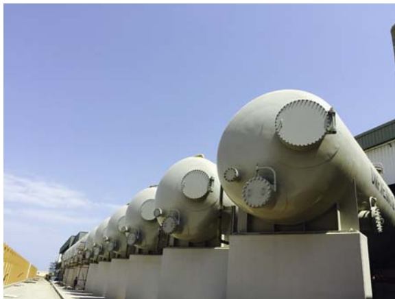
FIGURE 8.5 Horizontal pressure filters—Al-Ghubrah desalination plant, Oman.
