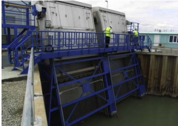
FIGURE 5.2 Coarse screens of onshore intake.
