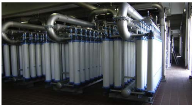
FIGURE 9.8 Pentair X-Flow Seaflex ultrafiltration pretreatment system.
