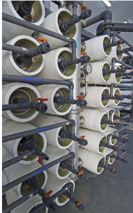
FIGURE 3.6 Membrane pressure vessel sampling ports.
