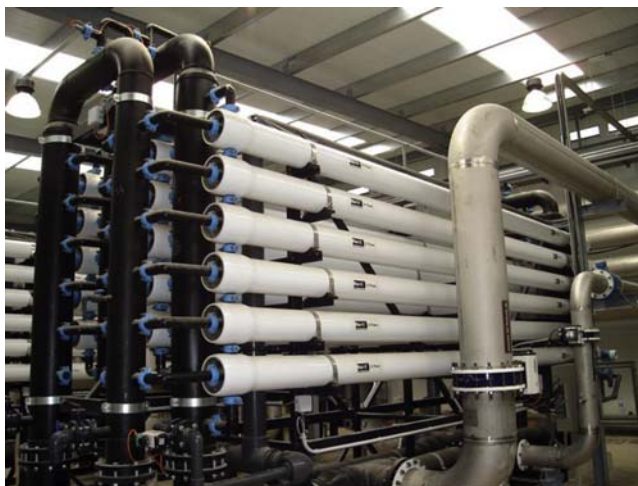
FIGURE 9.7 Pentair X-flow Seaguard ultrafiltration pretreatment system.
