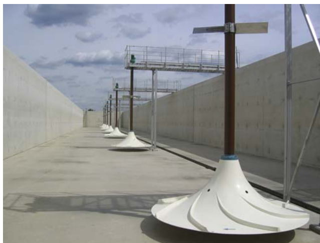
FIGURE 6.2 Flash mixers in coagulation tank.
