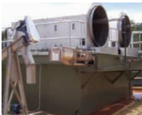
Solids Separation Module
